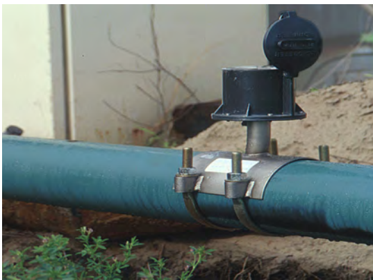
Figure 3.8. Field installation of a propeller meter.
