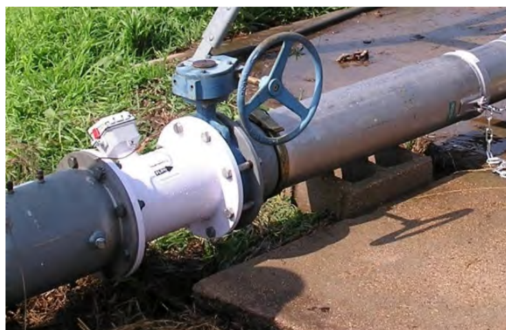
Figure 3.15. Electromagnetic flowmeter installed in the field.
