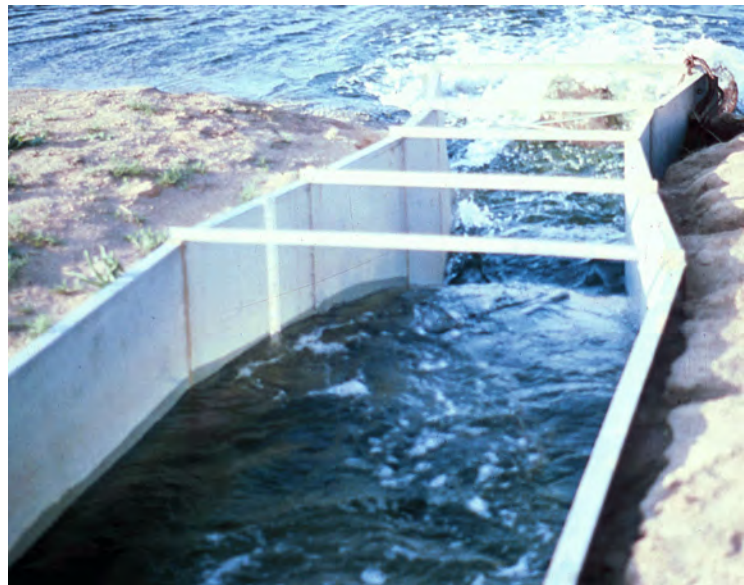
Figure 3.19. A Parshall flume to measure open channel flow.
