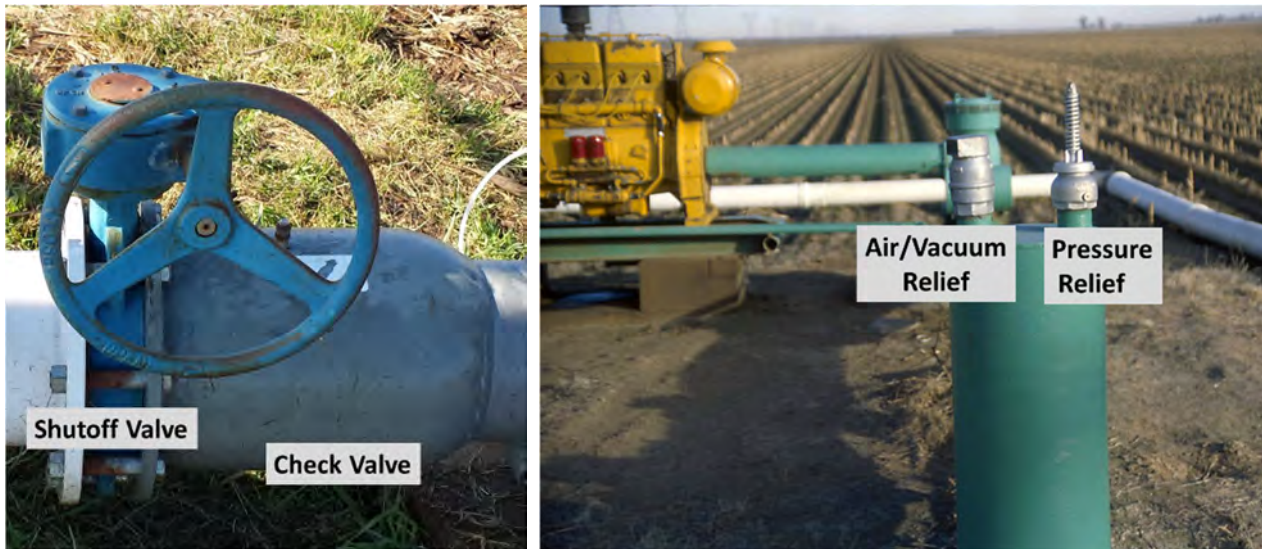
Figure 8.6. Irrigation pipeline protection valves.
