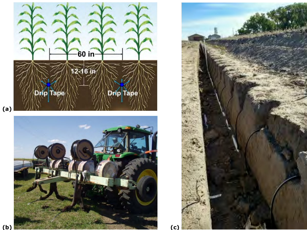
Figure 14.4. Installation of subsurface drip irrigation laterals: (a) schematic of a typical subsurface drip installation; (b) equipment for installing three subsurface drip laterals; and (c) laterals connected to the manifold. (Photos a and b courtesy of Suat Irmak, Nebraska Extension; photo c courtesy of Steve Melvin, Nebraska Extension.)
