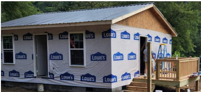
In-progress recovery efforts for homes via assistance from the Disaster Reconstruction Program.
