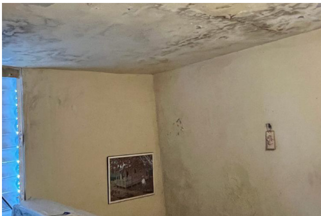
Extensive ceiling damage due to roof water leakages at Mrs. Carmen Burgos' home in Santa Isabel, Puerto Rico (pictured before repairs).
