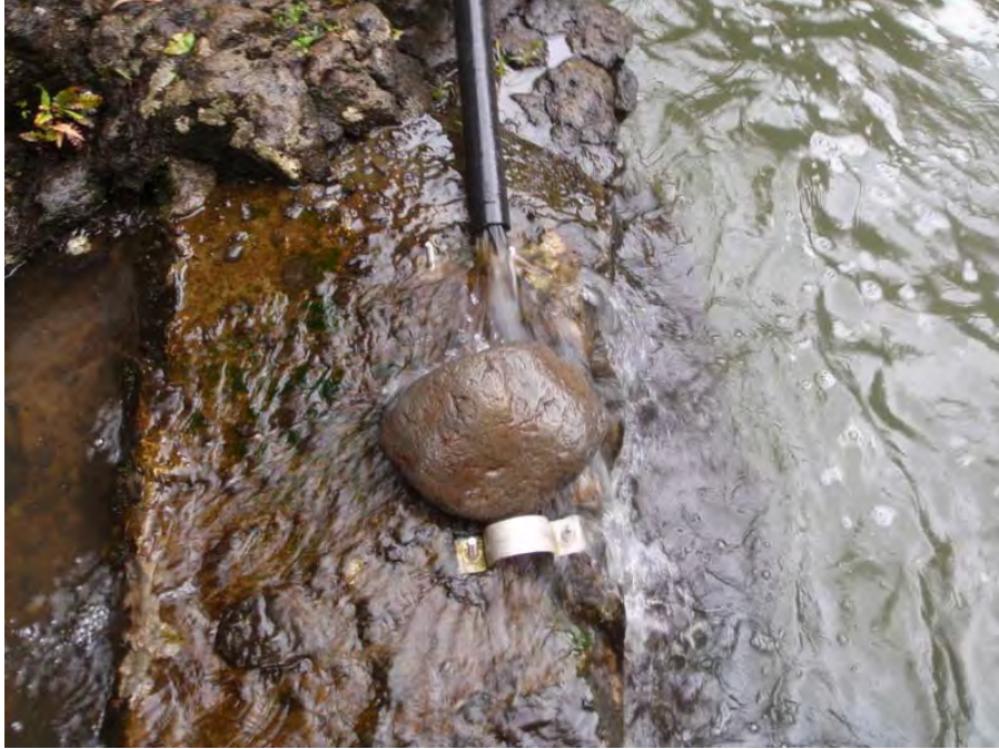
Water flowing over dam wall (gh002d-011p-041012)
