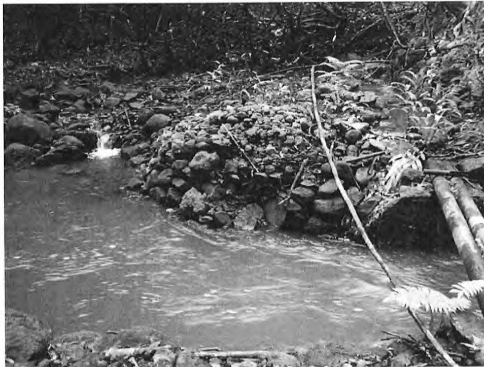
Note the two pipes on the right that pass over the ditch and transport water from stream. They are connected to one pvc pipe which empties back into the stream downstream.
