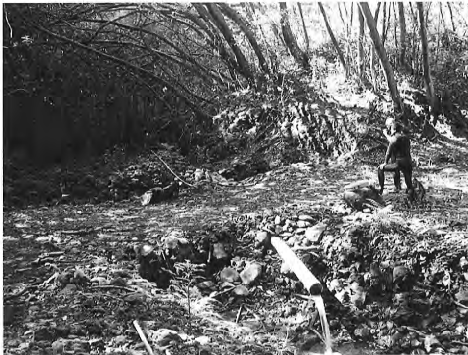
One pipe allowed to flow over irrigation ditch
