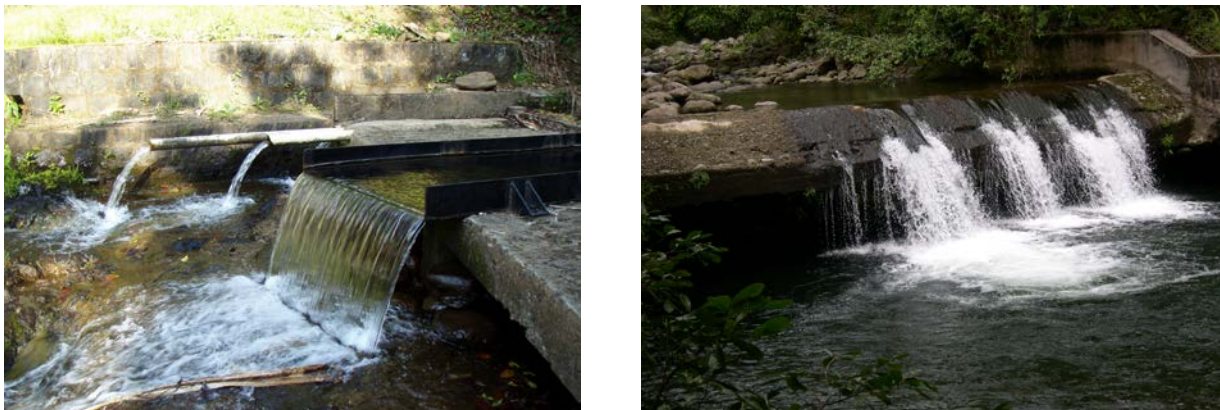
Figure 9. Over hanging diversions on Honopou Stream, Maui (left) and on the middle reach of Waihe‘e Stream, Maui (right). Notice how the water free falls and leaves no pathway for upstream migration.
