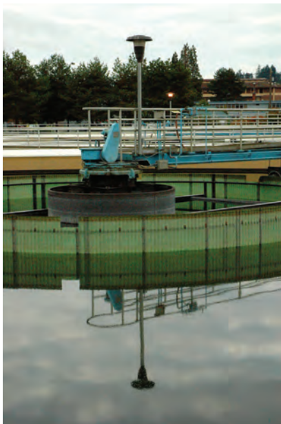
The LOTT sewage treatment plant in Olympia, Washington.
