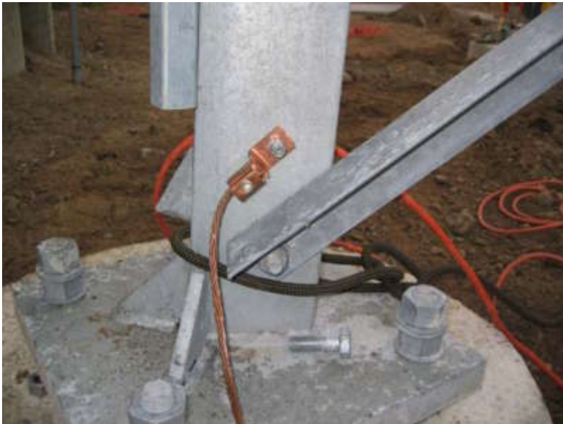
Figure 5.2: A tower with a heavy copper grounding wire.
