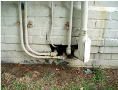
Utility conduits that provide entry points into a building include electrical lines or gas lines, TV cable or telephone lines, openings around water pipes, outdoor spigots, and water discharge lines from sump pumps. (Photo L. Pinto)
