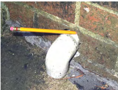
If a pencil fits under a door or into the space around a pipe, a young mouse could probably squeeze through, too. (Photo L. Pinto)
