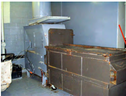
Rats or mice can live inside the block walls around a trash chute many floors up, and come down at night to feed in and around the compactor. (Photo L. Pinto)
