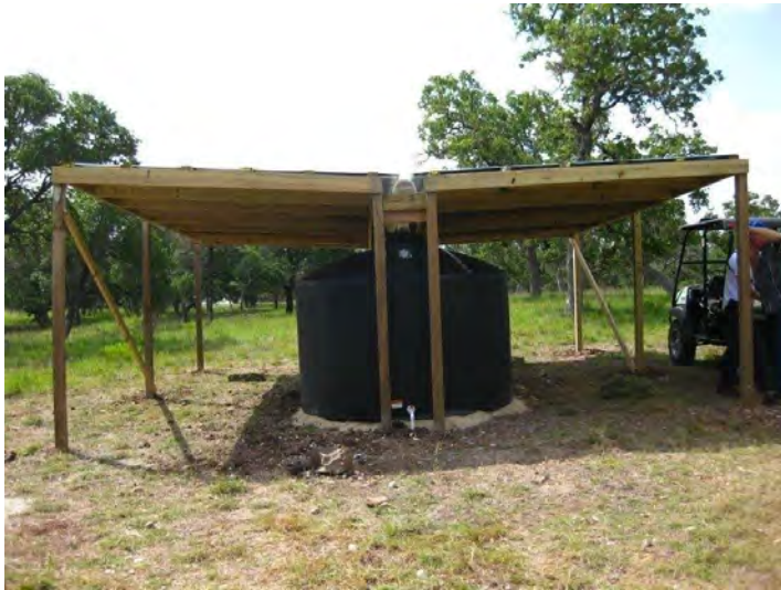
Above ground tanks
