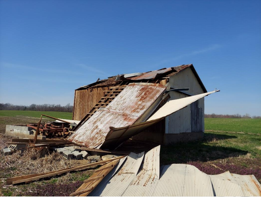
Photo: Storm Damage— Hans Schmitz (Purdue)
