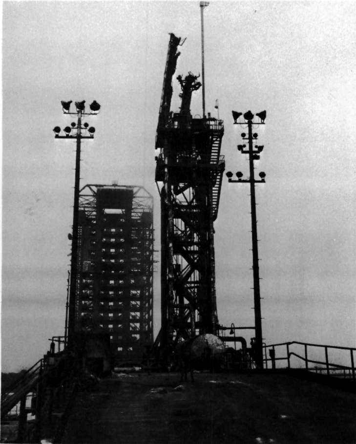
Figure XII-4. - View from ramp showing general damage to umbilical tower.
