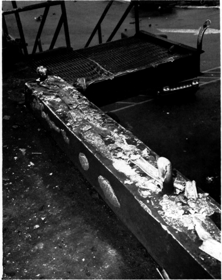
Figure XII-7. - View at top of ramp showing melted aluminum handrails and damage to grating.
