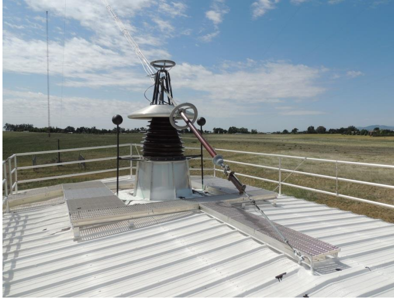
Fig. III.A.8. Roof of helix house and connection to antenna array.
