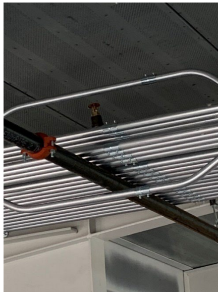
Figure 5-2. Conflict between Sprinkler Sprig and Electrical Conduit (Source: SEFT Consulting Group)
