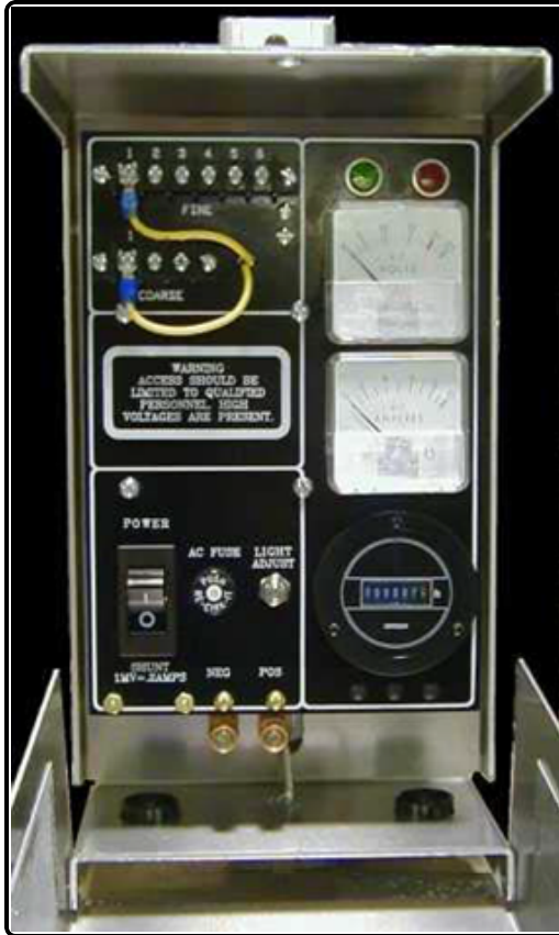
Impressed current rectifier
