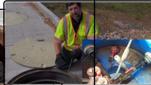
Submersible Turbine Pump Sump
