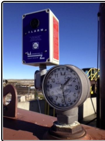
Overfill prevention alarm
