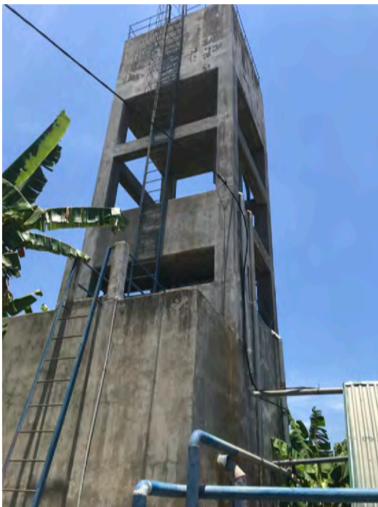
FIGURE 5. HA VINH WATER TREATMENT PLANT
