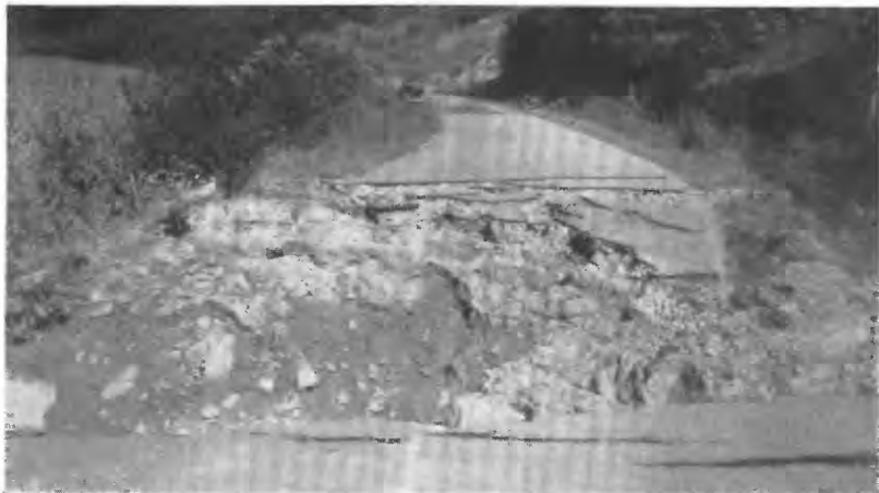
FIGURE 5.—Washed-out fill on State Route 5 at Jobs Run about 10 miles below Glenville. Courtesy of Corps of Engineers.
