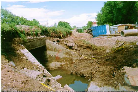
Figure 7. Failed culvert, 9:00 a.m. on the morning of 29 July 1997. Compacted dirt had all been washed away, and the 80 ft. long, 36 in. diameter pipe broken into pieces.
