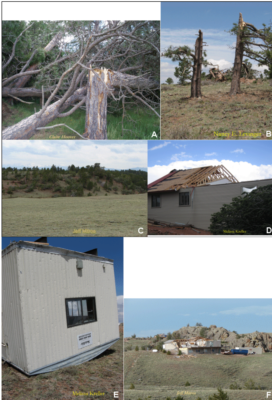
Figure 22(a-f). Storm damage photographs. Letters indicate location given on Fig. 21. Links to full resolution photos with credit: a) Claire Hoover, b) Nancy E. Levinger, c) Jeff Mitros, d) Melissa Kreller, e) Melissa Kreller, f) Jeff Mitros.
