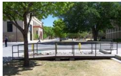
OFS recently rebuilt the Frenger footbridge, which spans a storm water drainage ditch adjacent to the International Mall.
