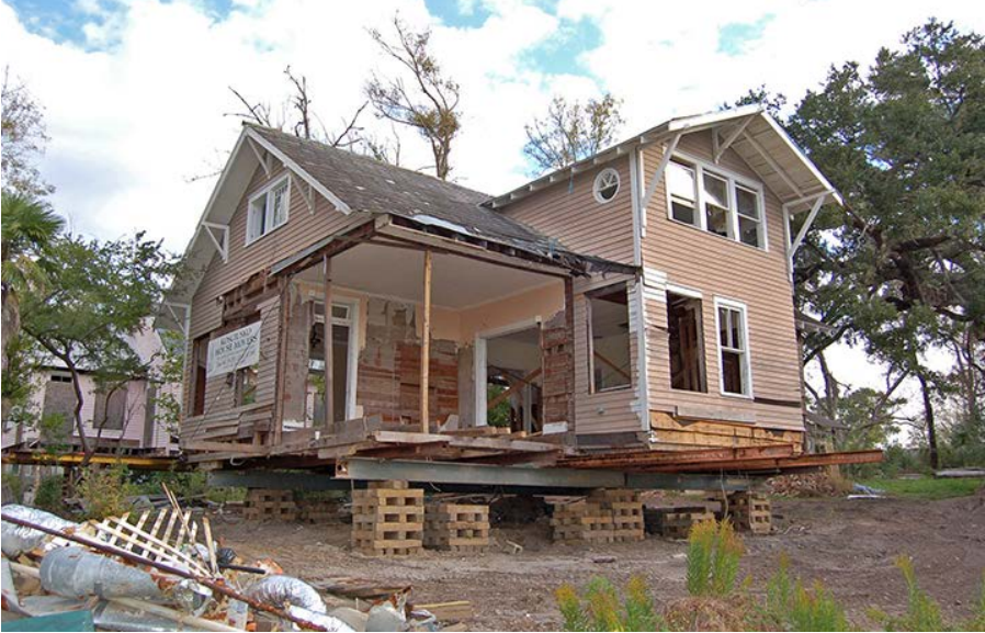
Many homes in Ocean Springs, Mississippi, were knocked off their foundations by Hurricane Katrina and had to be reset on piers during restoration.
