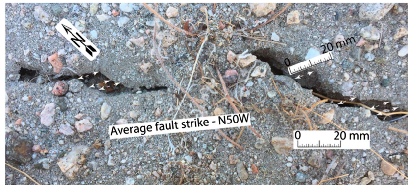
Figure 5. Example of an echelon surface rupture associated with creep event showing the small dilational steps used to measure displacement. Displacement in this example is estimated at 11 mm.
