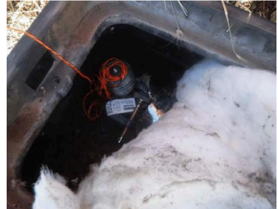
An installed leak detection sensor
