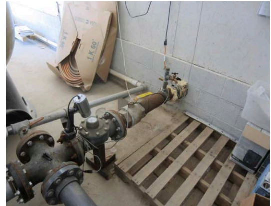
A flow monitor installed on the ABRA Water Company Water Pump
