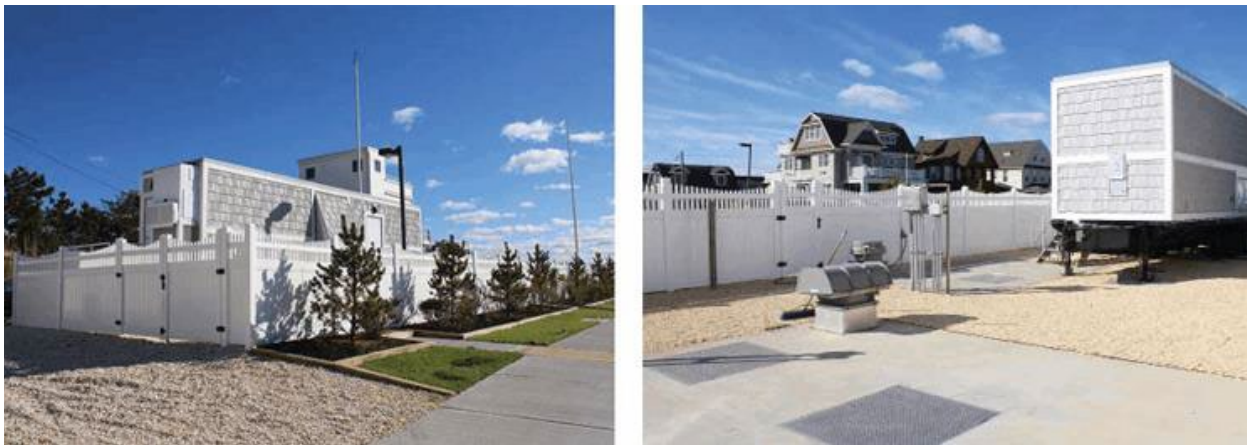
Figure 3. South Monmouth Regional Sewer Authority's second mobile pump station in the Borough of Belmar. Recognized by the Federal Emergency Management Agency (FEMA) and the EPA as 'Best Management Practice' for mitigation of damages related to extreme wet weather events (Dalal, 2017).
