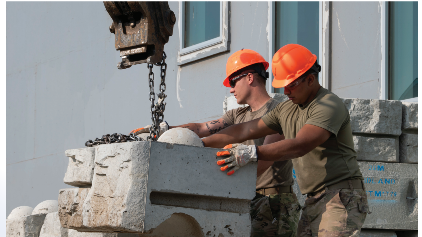
U.S. Air Force Senior Airmen Shane Baumann and Mitchell Terrell, assigned to the 307th Civil Engineer Squadron, build a retaining wall for a regional science, technology, engineering, and mathematics center in Woodbine, Iowa, June 16, 2023. The building was a Department of Defense Innovative Readiness Training initiative for Ignite Pathways, an educational nonprofit group. IRT missions help communities and nonprofits while providing essential training for U.S. military personnel. (U.S. Air Force Photo by Airman 1st Class Justin Moore)
