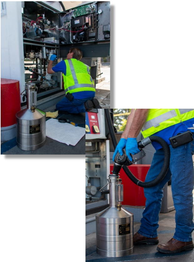
Photos 8 and 9: RSA making repairs to gas dispenser; after the repair it is tested using a certified standard (prover)
