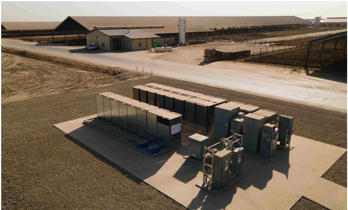
Image 55. Fuel cells at Bar 20 Dairy.
