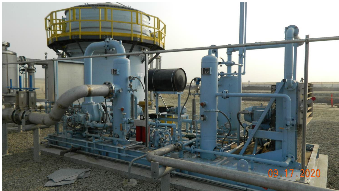
Image 22. Gas compressor equipment at BV Dairy.
