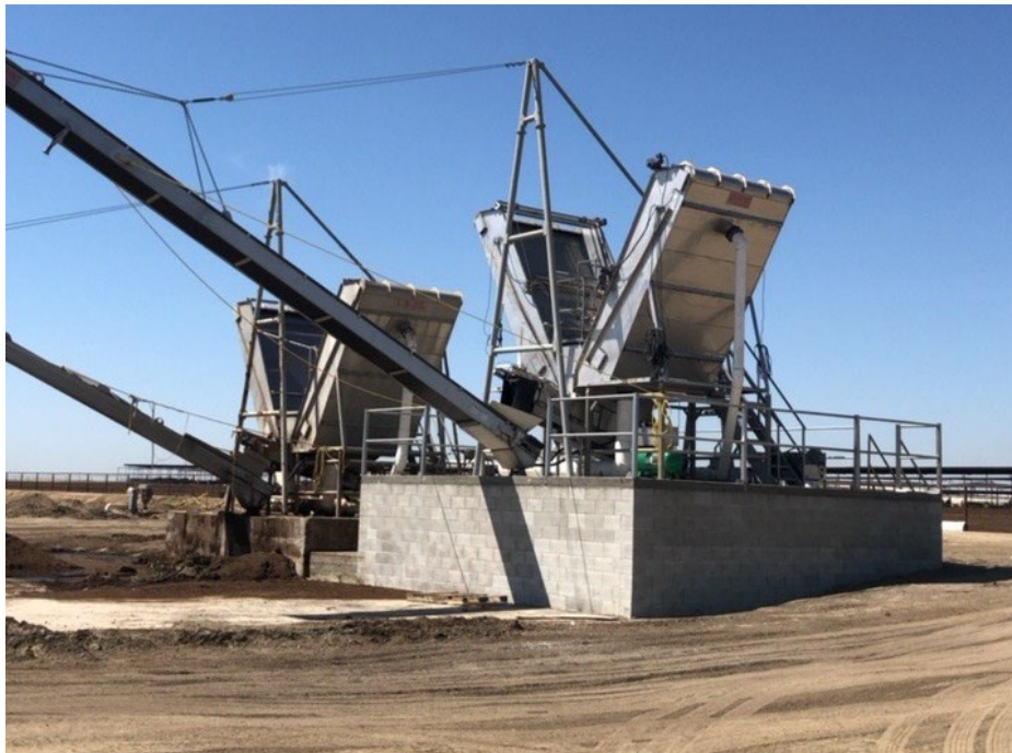
Image 50. New solid separators at Scheenstra Dairy.
