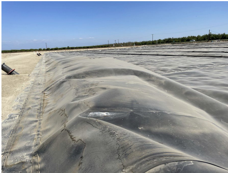
Image 45. Close up of the new covered lagoon digester at Rancho Sierra Dairy.
