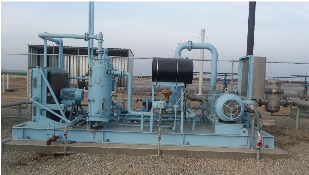
Image 27. Biogas compressor skid at Western Sky Dairy.
