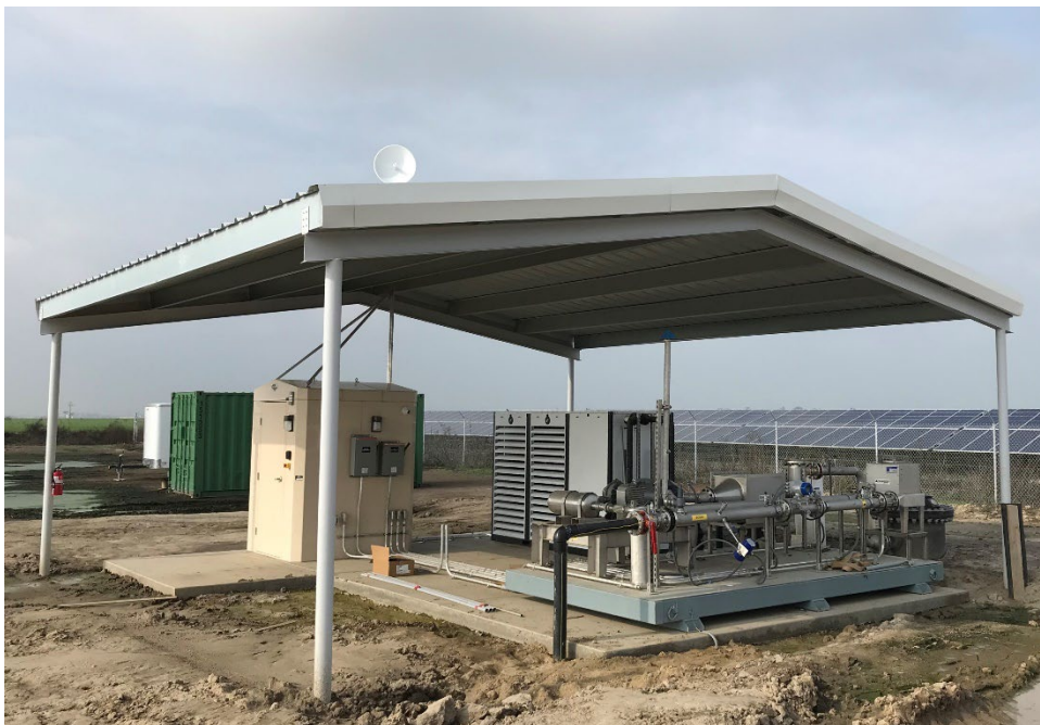
Image 17. Biogas conditioning equipment at Little Rock Dairy.
