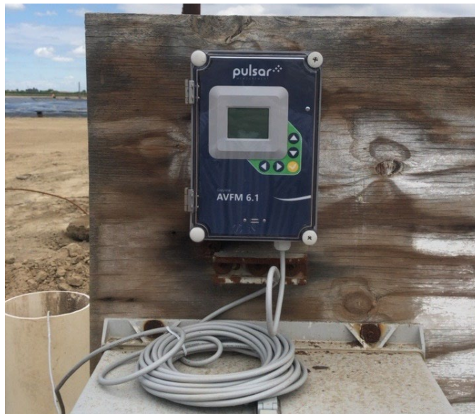
Image 48. Digester wastewater flowmeter at Bos Farms Dairy.
