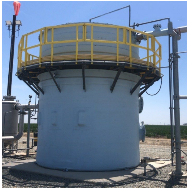
Image 42. H 2 S scrubber at Wreden Ranch Dairy.
