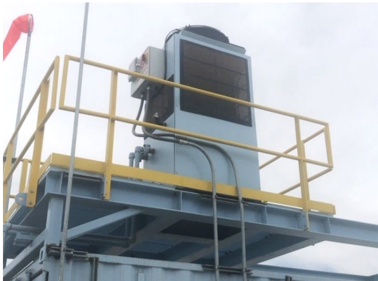
Image 34. Chillers in the biogas conditioning skid at Aukeman Dairy.
