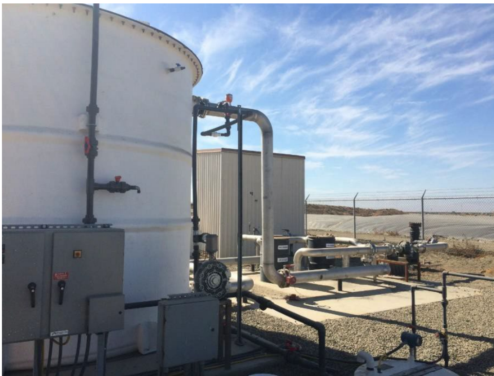
Image 2. A view of the Open Sky Ranch Dairy digester.
