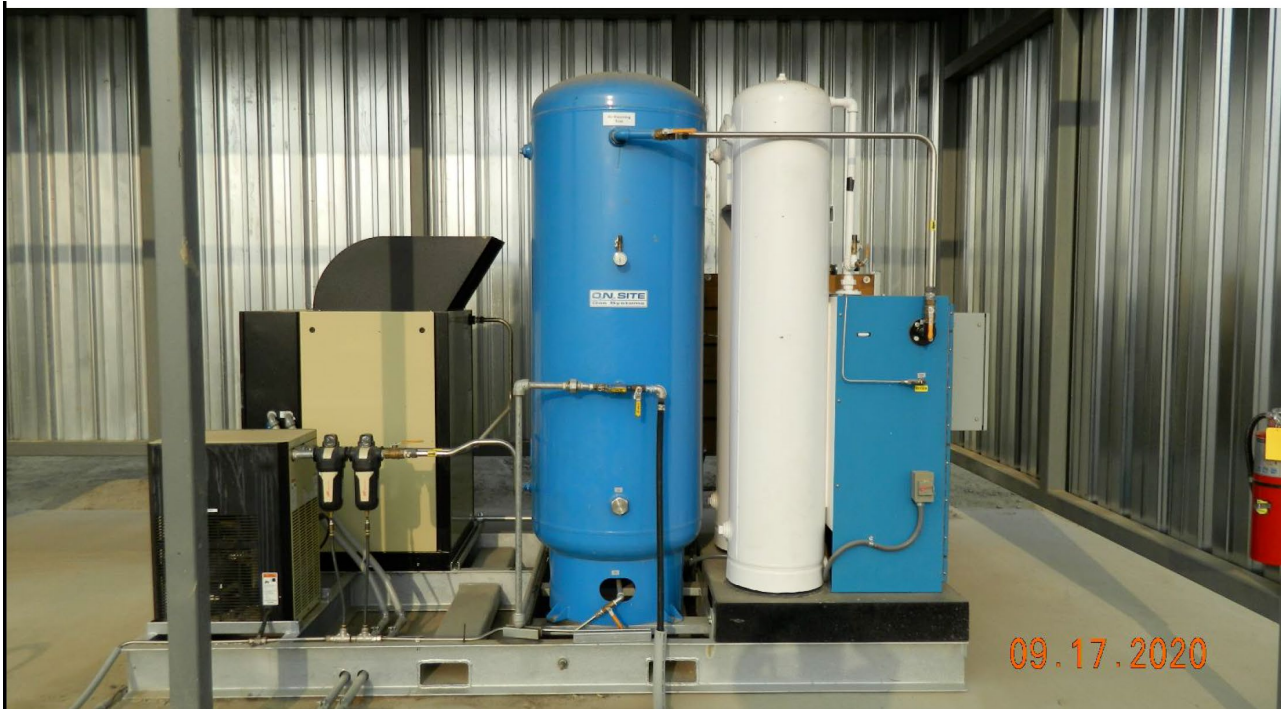
Image 19. An oxygen generator skid for biological control of hydrogen sulfide (H 2 S) at Trilogy Dairy.
