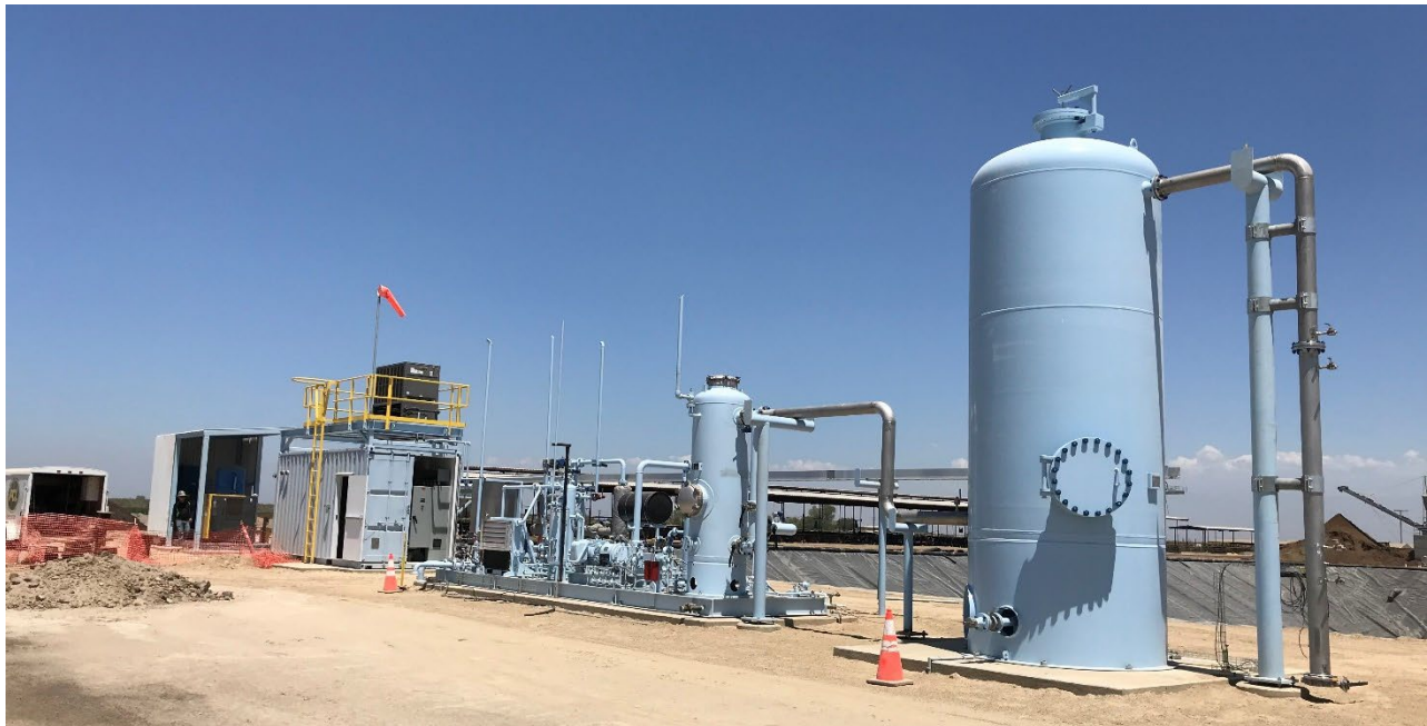
Image 56. Biogas conditioning equipment at Ribeiro Dairy.
