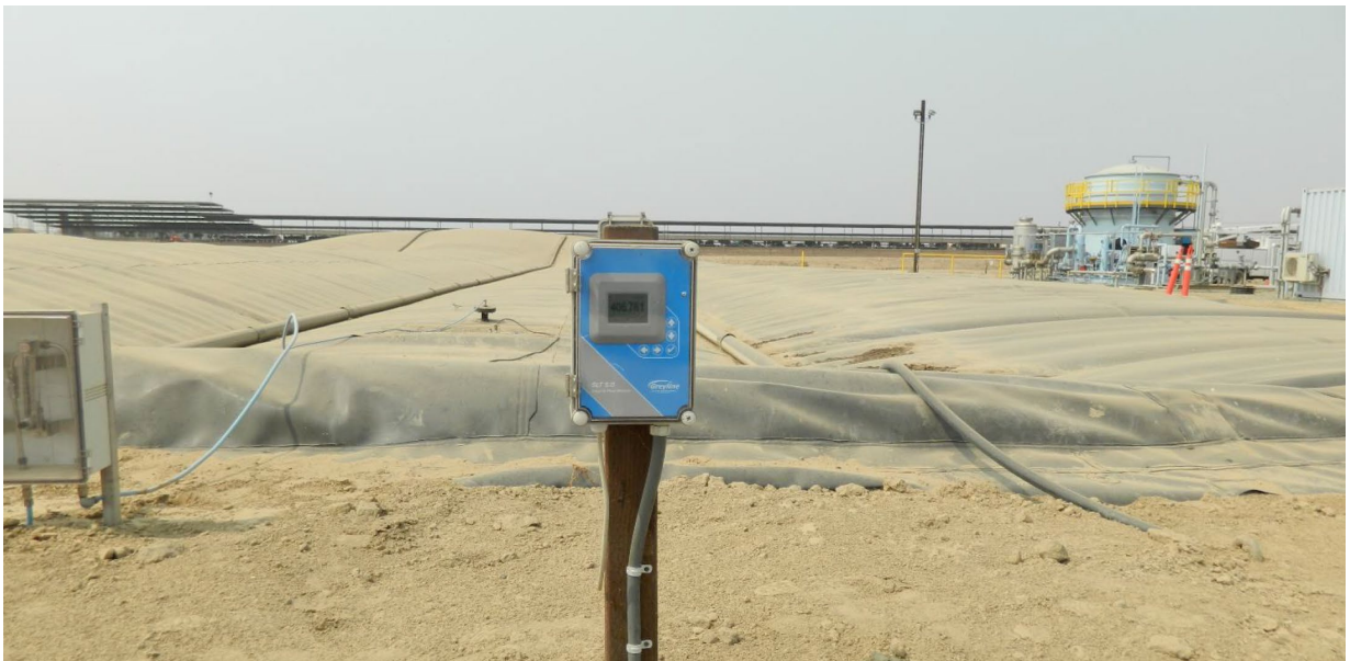
Image 18. Weir box and a weir box meter (foreground) and covered lagoon digester and biogas conditioning equipment (background) at Maple Dairy.
