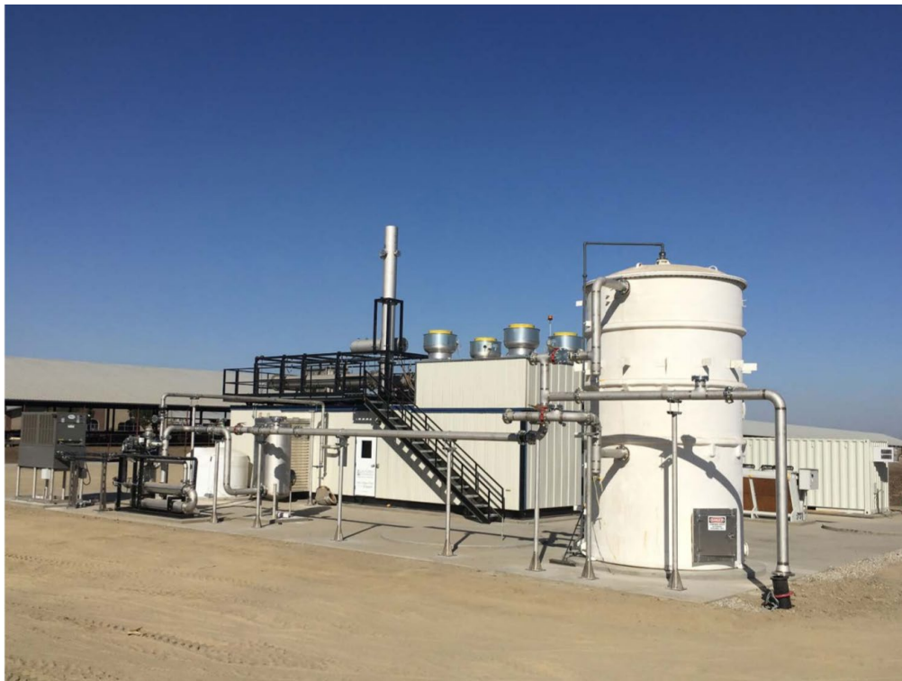
Image 7. Electric generation equipment at the Carlos Echeverria & Sons Dairy Biogas Project.
