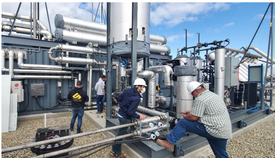
Image 28. Biogas conditioning system at FM Jerseys Dairy
