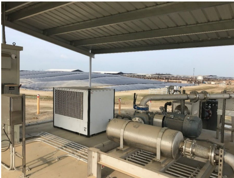
Image 15. Biogas conditioning equipment (foreground) and covered lagoon digester (background) at Riverview Dairy.
