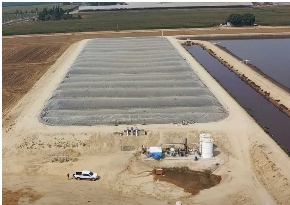
Image 23. Aerial view of the covered lagoon digester and the biogas conditioning equipment at Double D Dairy.
