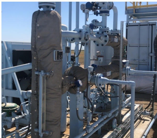
Image 35. Dehydration skid at Dykstra Dairy.
