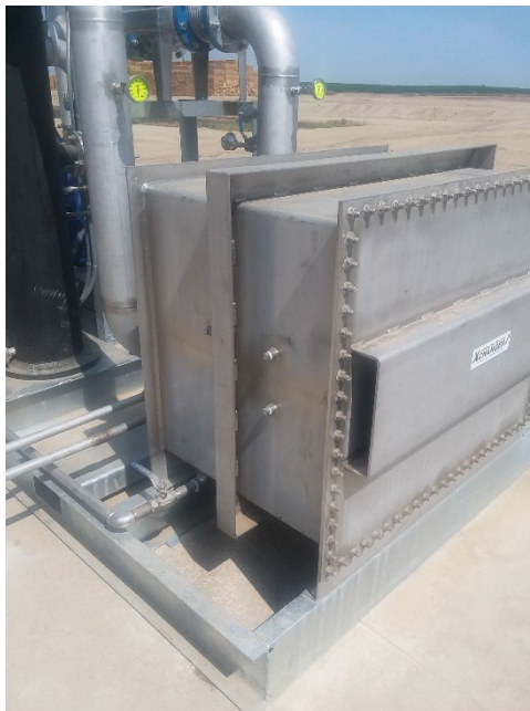
Image 54. Heat exchanger equipment at Belonave Dairy.
