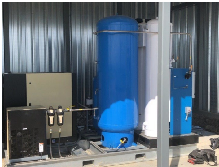
Image 43. Oxygen and air compressor at Valadao Dairy.
