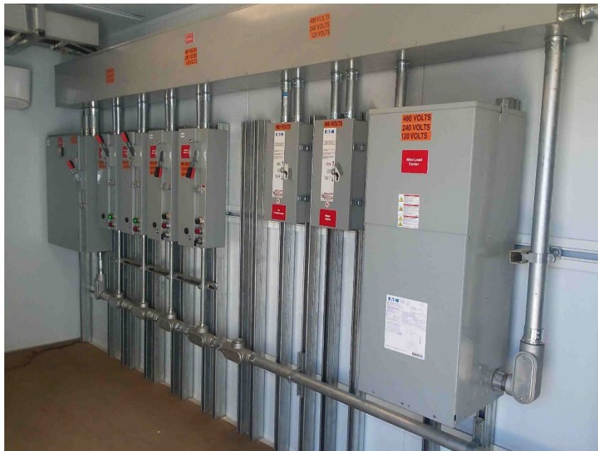
Image 44. Power Distribution Center room at Jacobus De Groot #2 Dairy.
