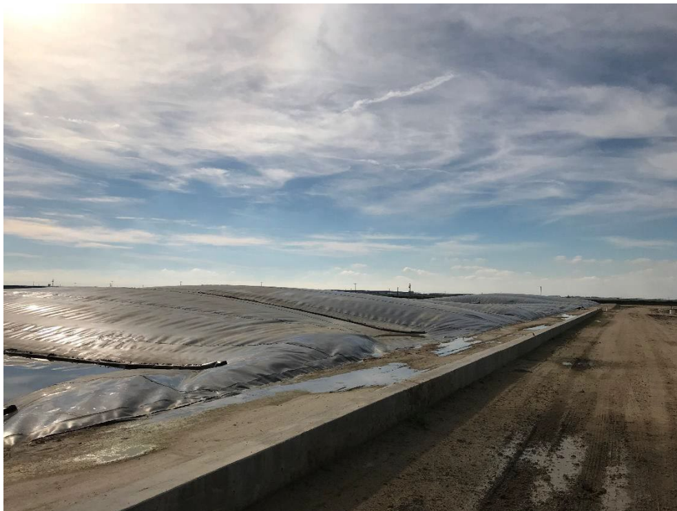
Image 9. Covered lagoon digester at R Vander Eyk Dairy
