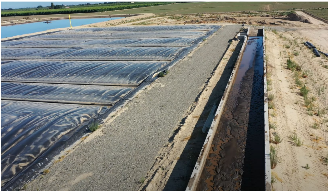
Image 21. Sand lane and covered lagoon digester at Ackerman Dairy.
