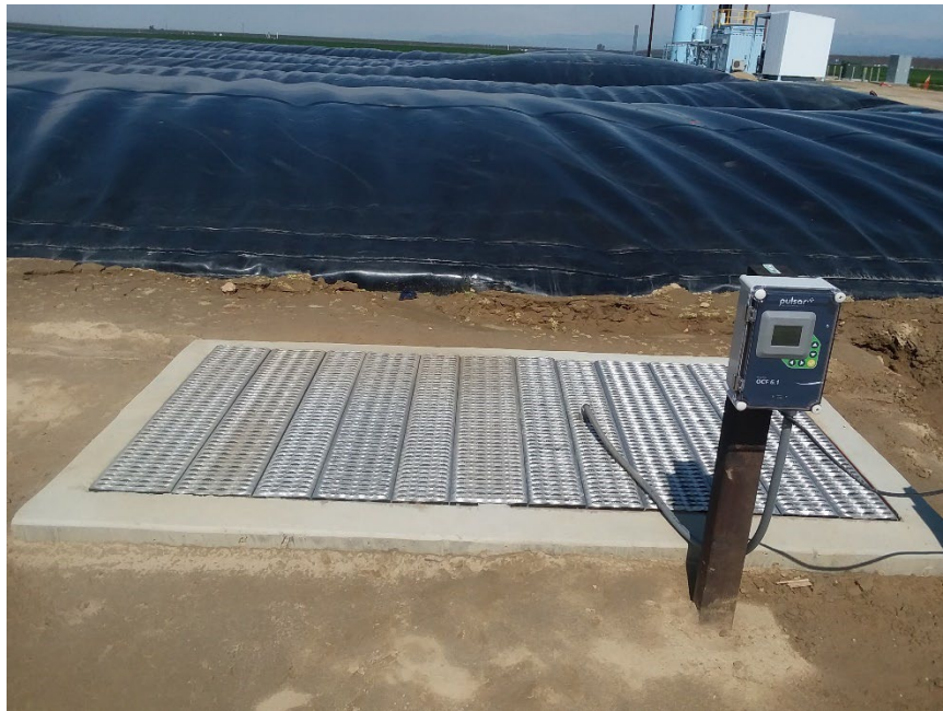
Image 33. Weir box and new covered lagoon digester at Rob Van Grouw Dairy.
