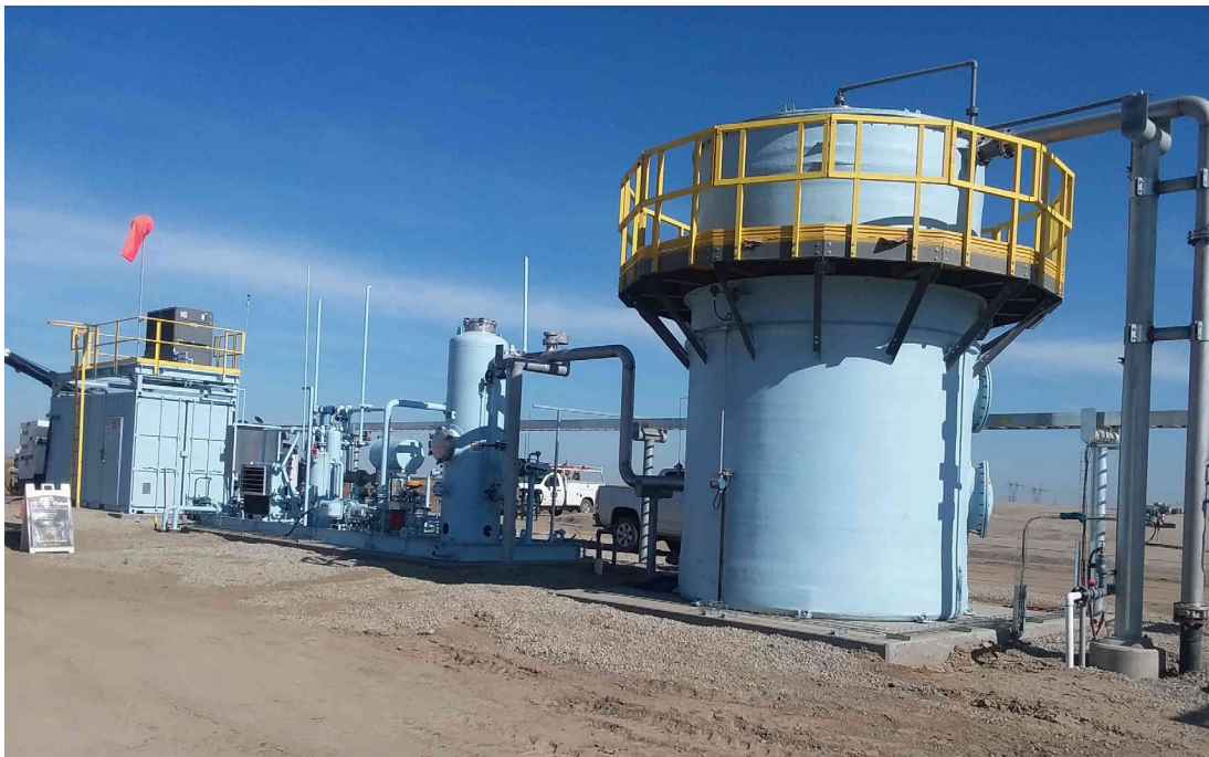
Image 53. Biogas conditioning equipment at Newhouse Dairy.
