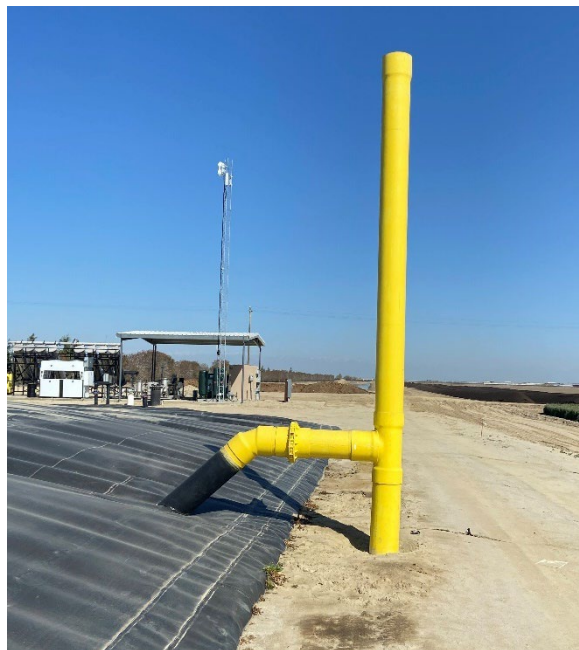
Image 29. Emergency vent stack at River Ranch Dairy Digester Pipeline Project.
