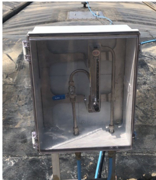
Image 41. Oxygen rotameter in a covered dairy digester at Hollandia Dairy.
