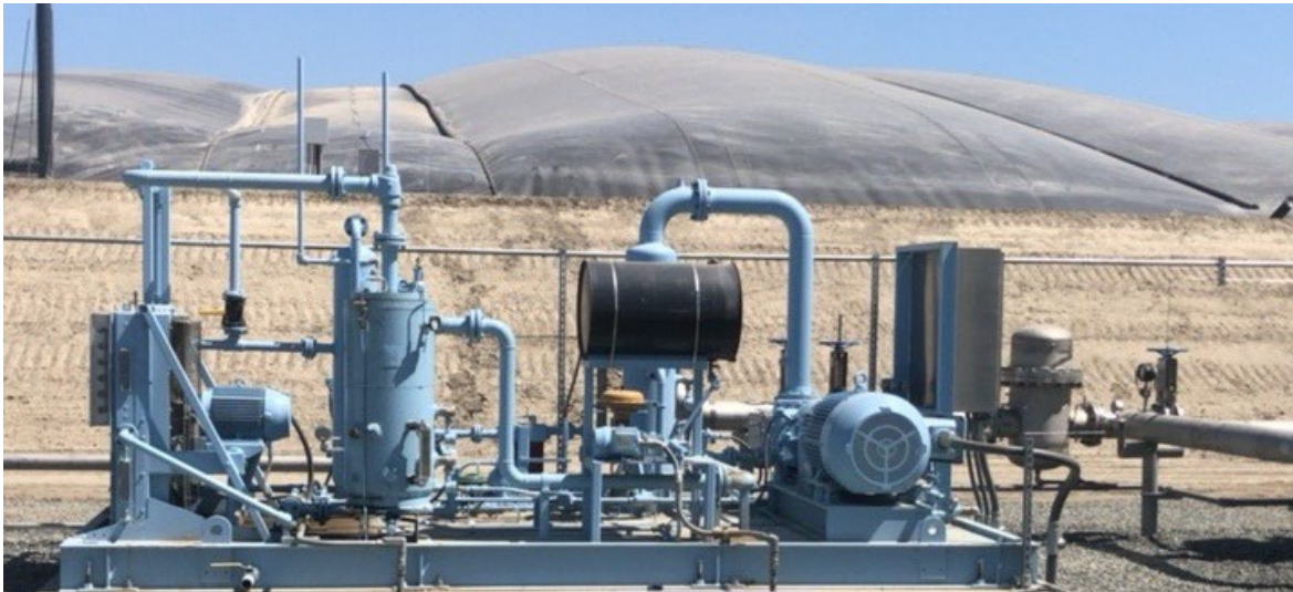
Image 40. Gas compressor equipment at Cloverdale Dairy.
