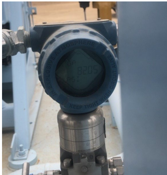
Image 46. Biogas flowmeter at Rancho Teresita Dairy.
