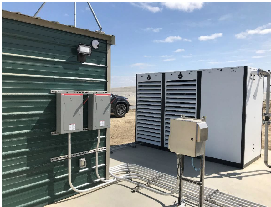
Image 11. Biogas conditioning equipment (foreground) and covered lagoon digester (background) at Cornerstone Dairy.
