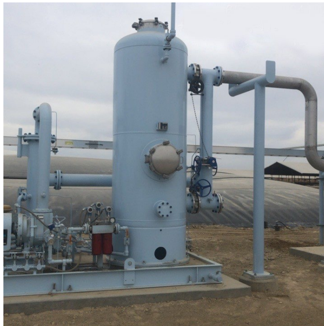
Image 47. Activated carbon vessel at Riverbend Dairy.
