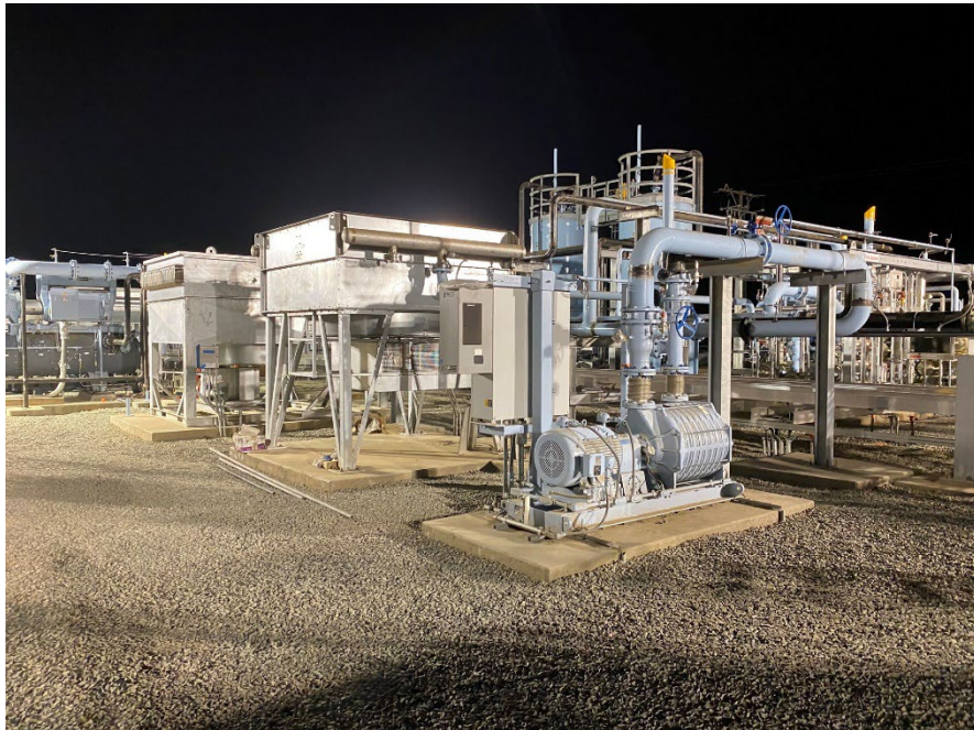
Image 24. Upgrader equipment at the CalBioGas West Visalia Cluster, which receives biogas from S&S Dairy.
