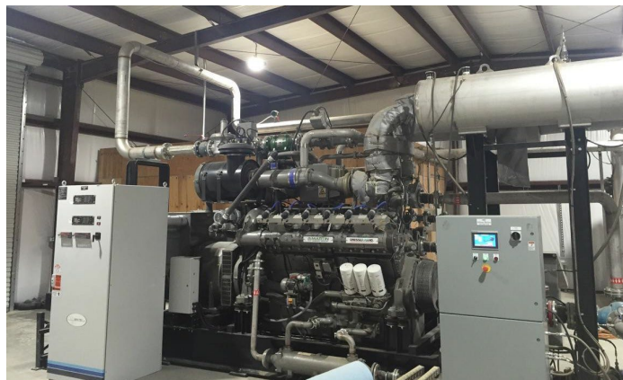
Image 4. Installed electrical genset at Verwey-Madera Dairy.
