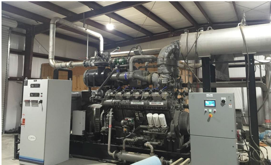
Image 6. Installed electrical genset at Verwey-Madera Dairy.
