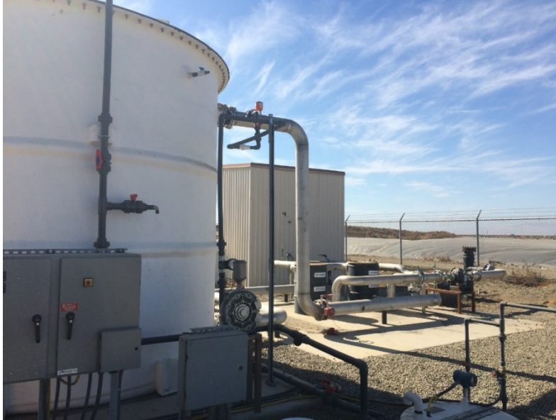
Image 4. A view of the Open Sky Ranch Dairy digester.
