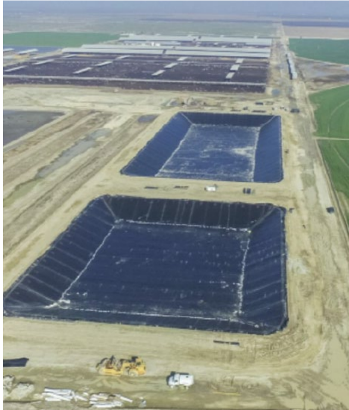
Image 7. Aerial view of West-Star North Dairy Digester
