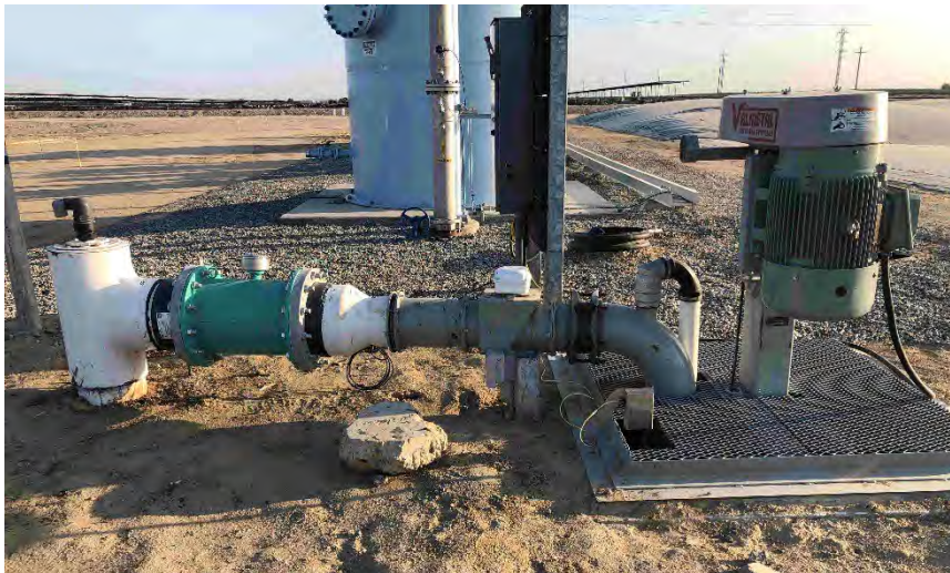
Image 73. Irrigation vault and meter at Southern Cross Dairy.
