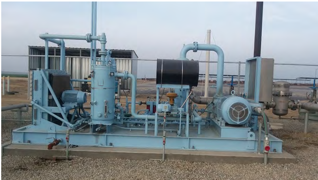
Image 27. Biogas compressor skid at Western Sky Dairy.
