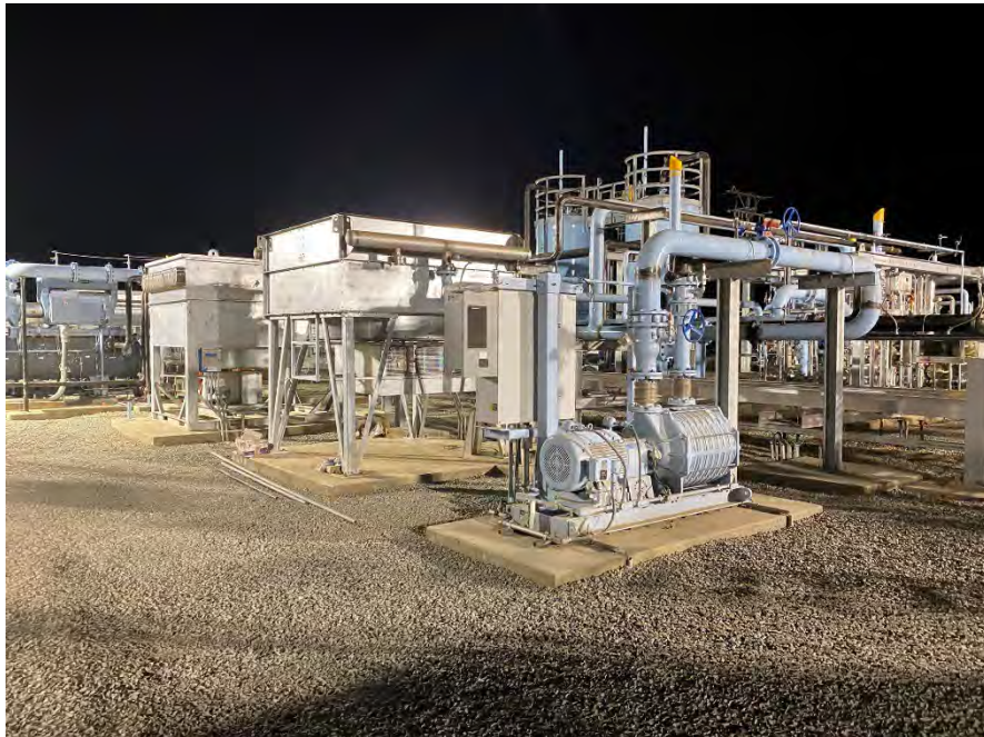
Image 24. Upgrader equipment at the CalBioGas West Visalia Cluster, which receives biogas from S&S Dairy.
