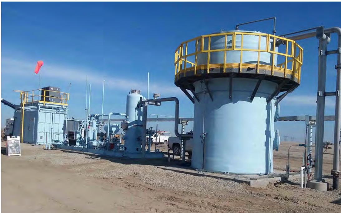
Image 53. Biogas conditioning equipment at Newhouse Dairy.
