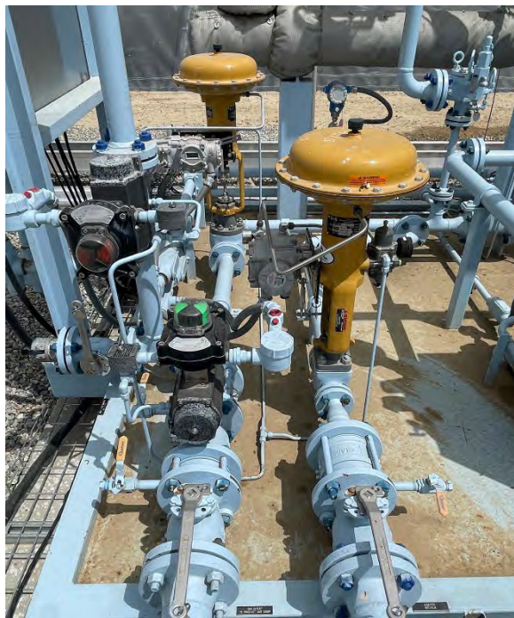
Image 67. Metering skid at Whiteside Dairy.
