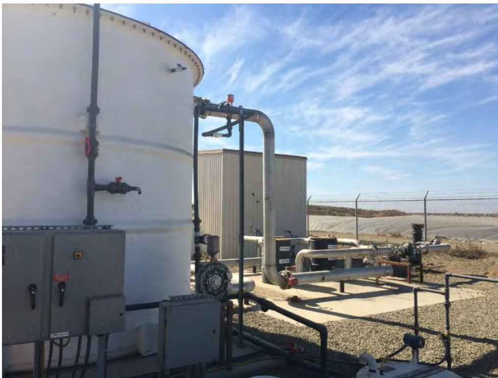
Image 2. A view of the Open Sky Ranch Dairy digester.
