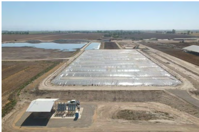
Image 77. New covered lagoon digester and conditioning skid at Hoogendam Dairy.
