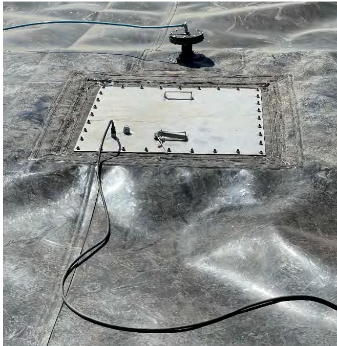
Image 37. Mixer and oxygen port in the covered lagoon
