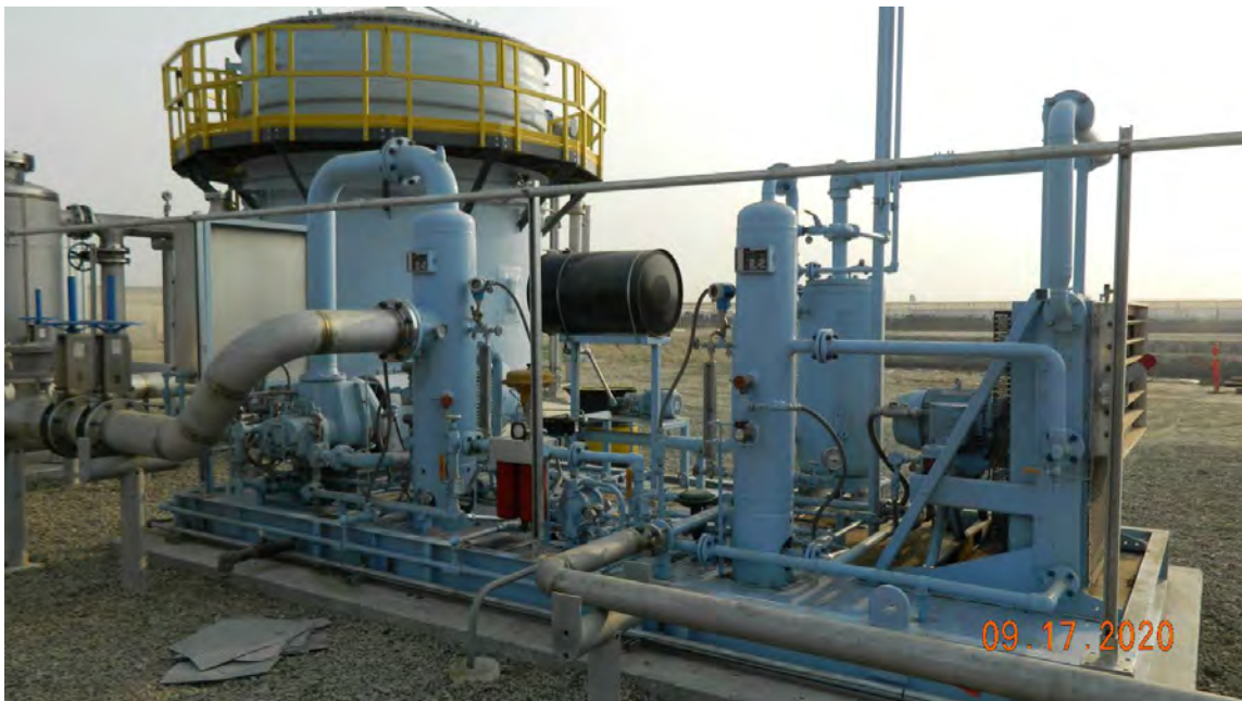
Image 22. Gas compressor equipment at BV Dairy.
