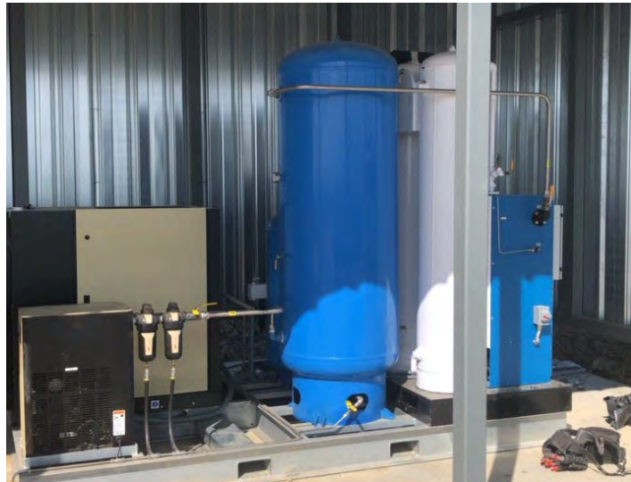
Image 43. Oxygen and air compressor at Valadao Dairy.
