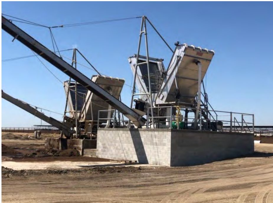
Image 50. New solid separators at Scheenstra Dairy.
