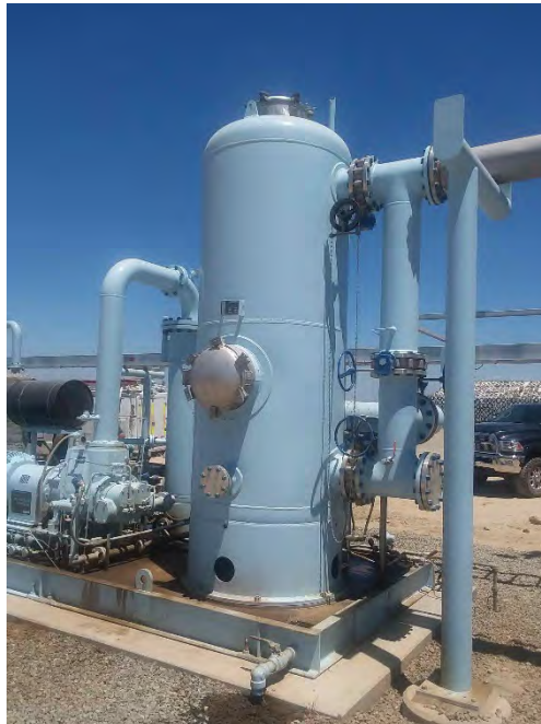
Image 32. Activated Carbon Vessel at Double J Dairy.
