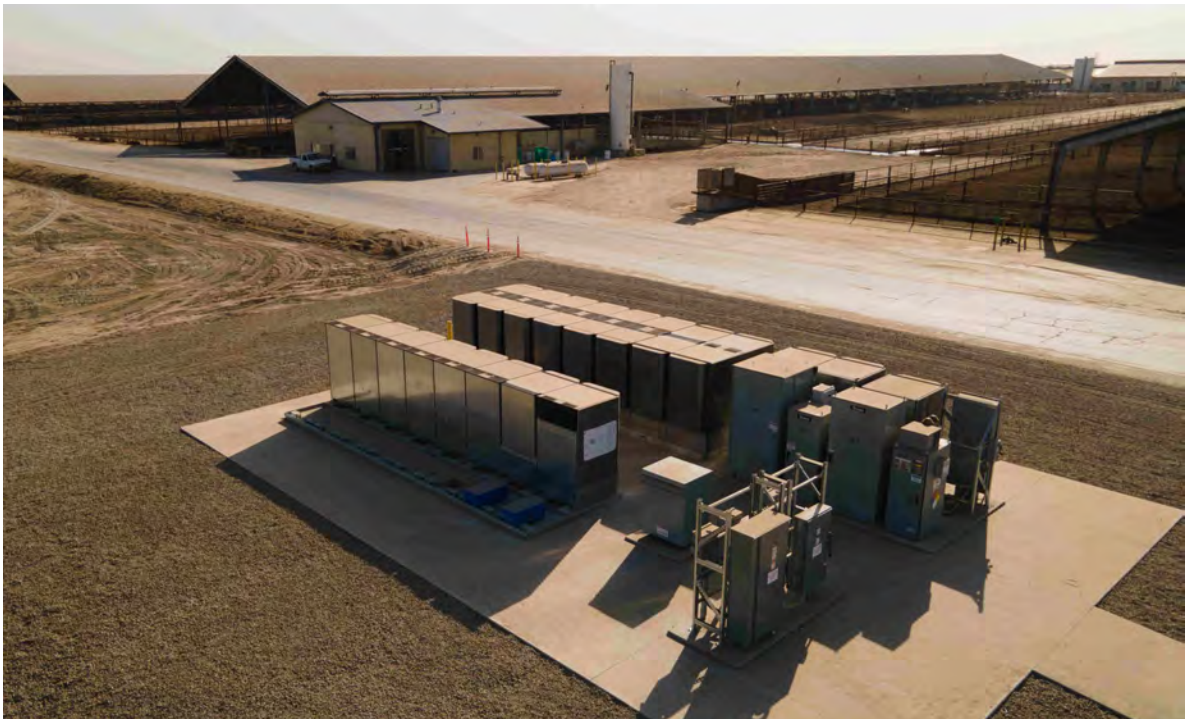
Image 56. Fuel cells at Bar 20 Dairy.
