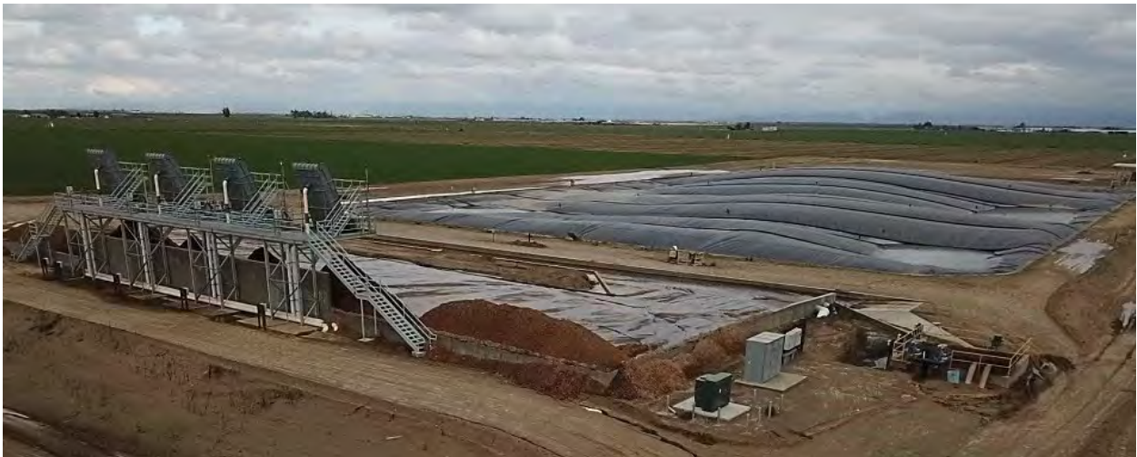
Image 57. New covered lagoon digester at Hettinga Centralized Dairy.
