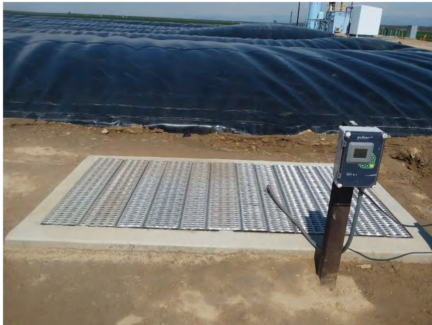
Image 33. Weir box and new covered lagoon digester at Rob Van Grouw Dairy.
