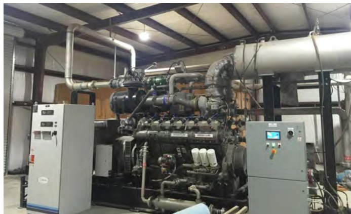
Image 4. Installed electrical genset at Verwey-Madera Dairy.
