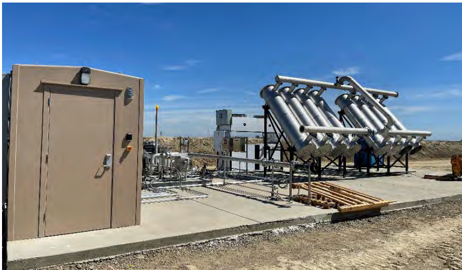
Image 64. Biogas conditioning equipment at Red Rock Dairy.
