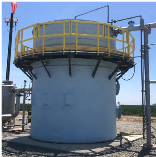
Image 42. H 2 S scrubber at Wreden Ranch Dairy.
