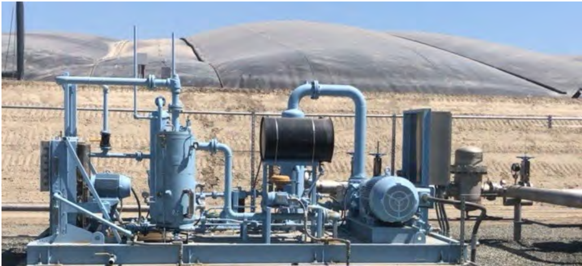
Image 40. Gas compressor equipment at Cloverdale Dairy.
