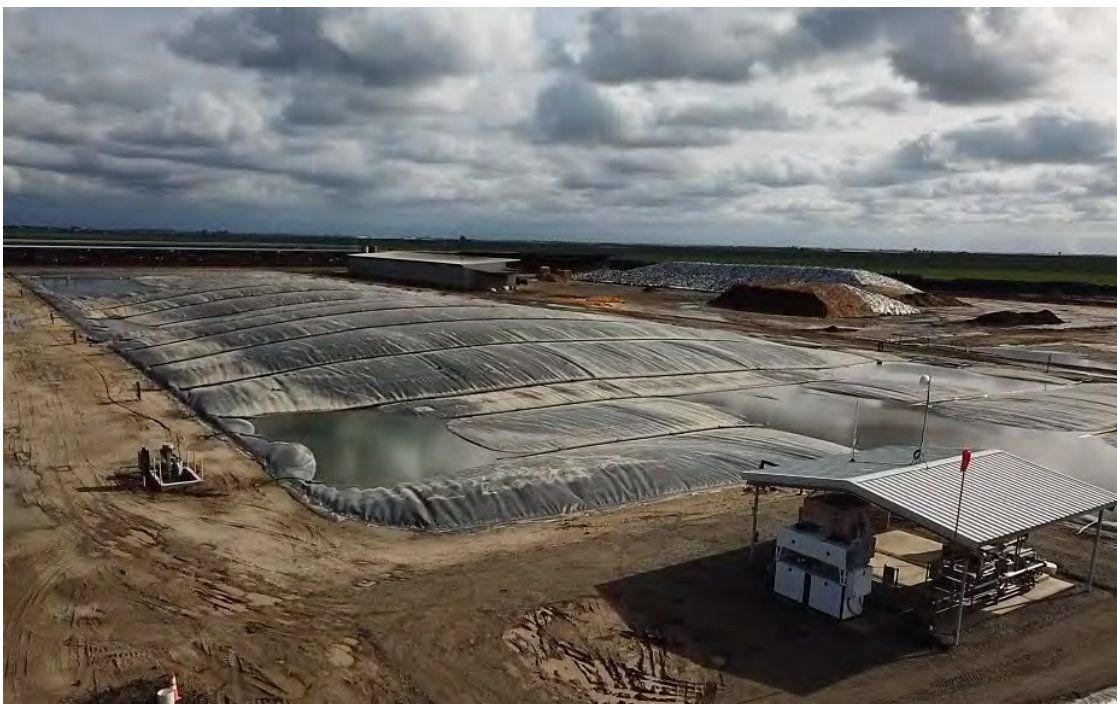
Image 60. New covered lagoon digester at Pixley Dairy.
