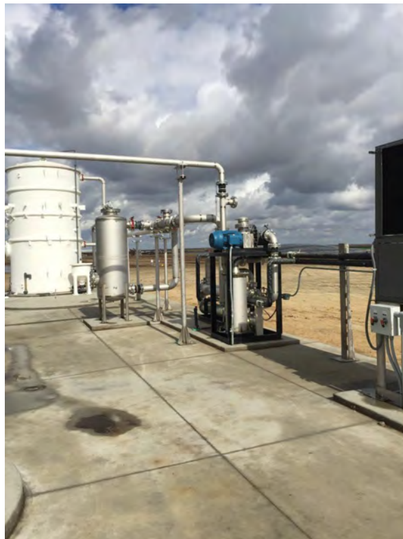
Image 5. Biogas conditioning and electric generation equipment (foreground) with covered lagoon digester (background) at the West-Star North Dairy.
