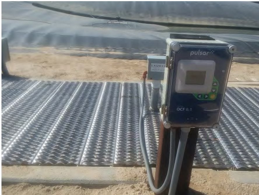
Image 66. Weir box and wastewater flowmeter at Skyview Dairy.
