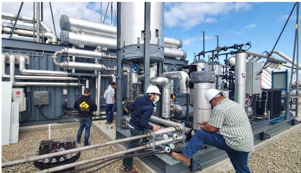
Image 28. Biogas conditioning system at FM Jerseys Dairy
