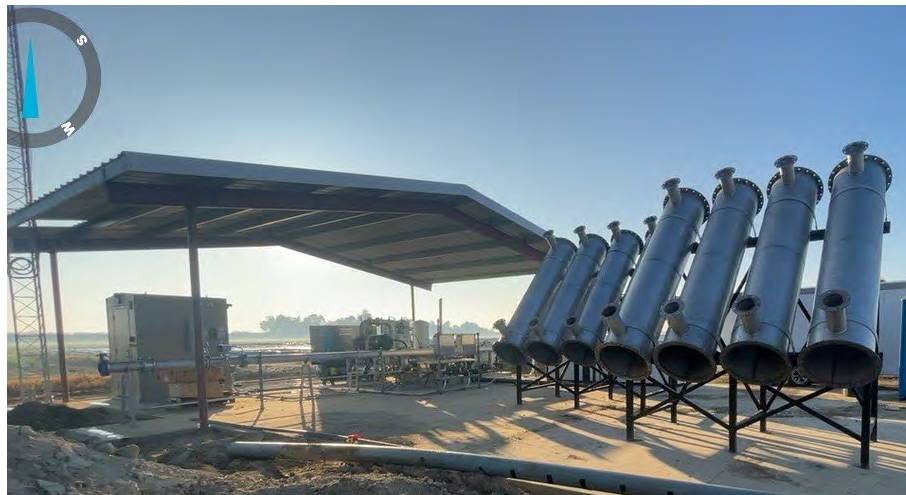
Image 78. Biogas conditioning skid at Double Diamond Dairy.
