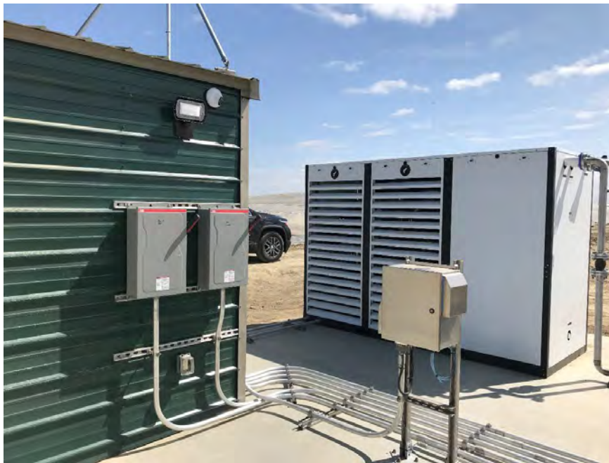
Image 11. Biogas conditioning equipment (foreground) and covered lagoon digester (background) at Cornerstone Dairy.
