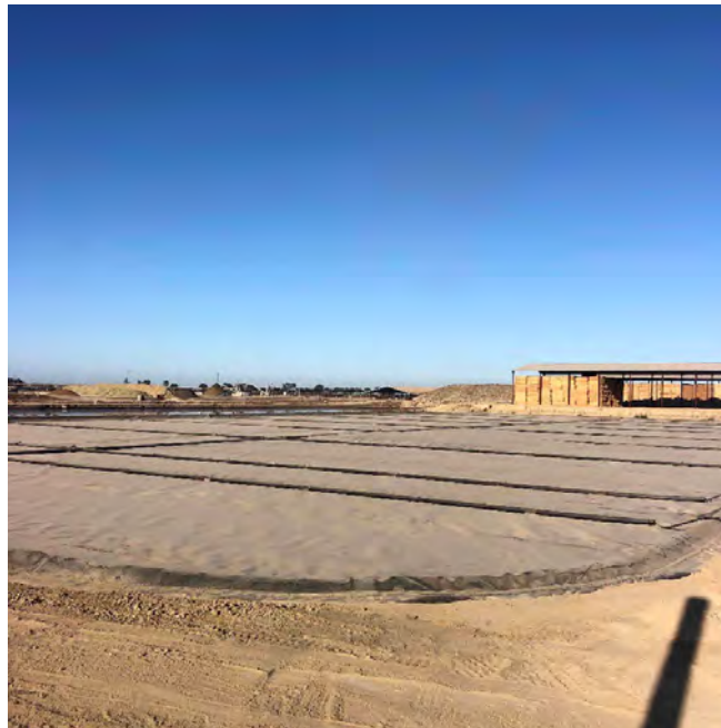
Image 26. Covered lagoon digester at Hamstra Dairy.
