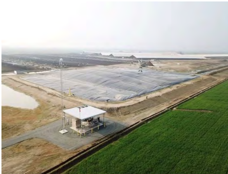
Image 54. New covered lagoon digester at Northstar Dairy.
