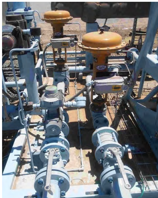
Image 38. Metering equipment at Mineral King Dairy.
