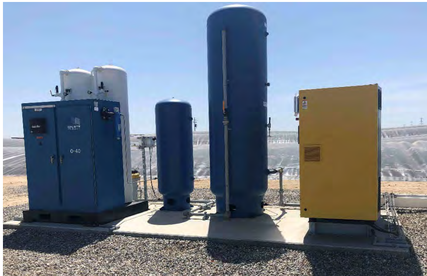
Image 72. Oxygen and air compressor skid at Maya Dairy.
