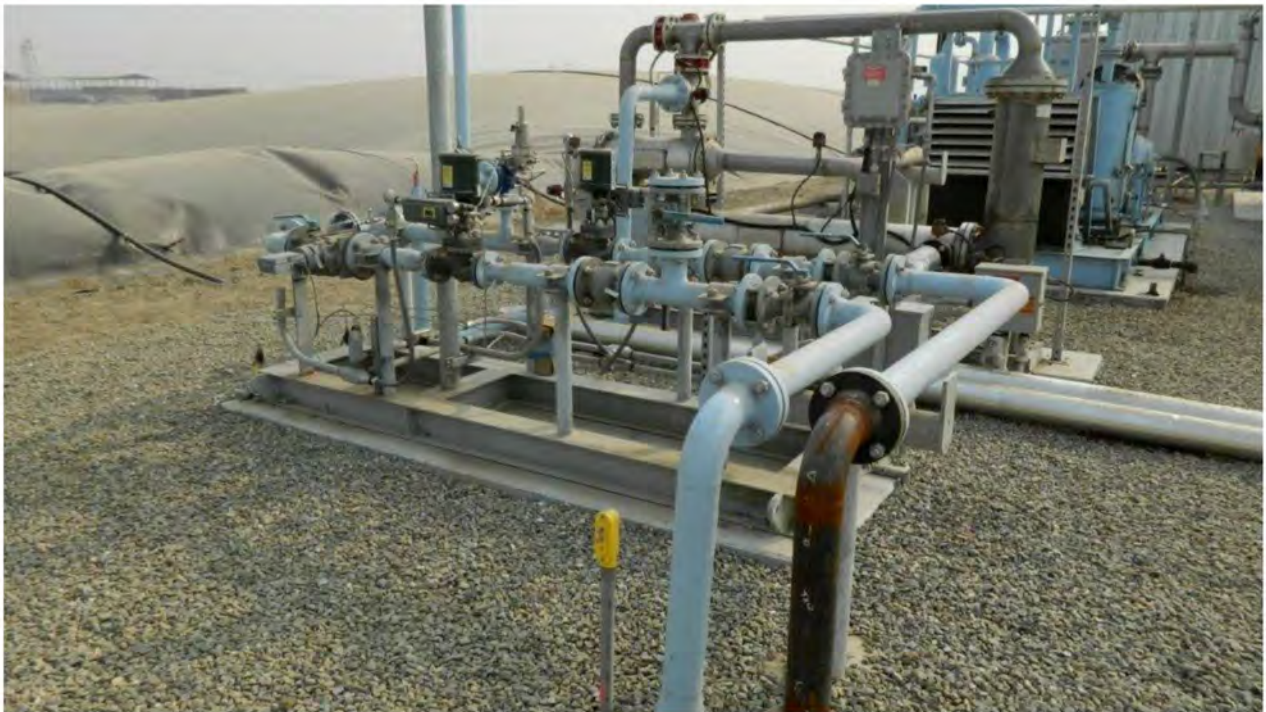
Image 20. Gathering line array (foreground) and covered lagoon digester (background) at T&W Dairy.
