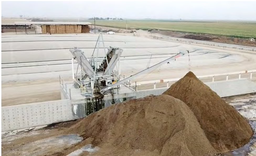
Image 81. Mechanical solid separator at Simoes Centralized Digester Project.
