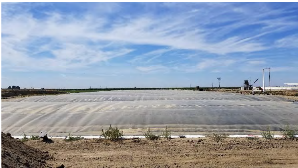
Image 12. Covered lagoon dairy digester at Sousa & Sousa Dairy.
