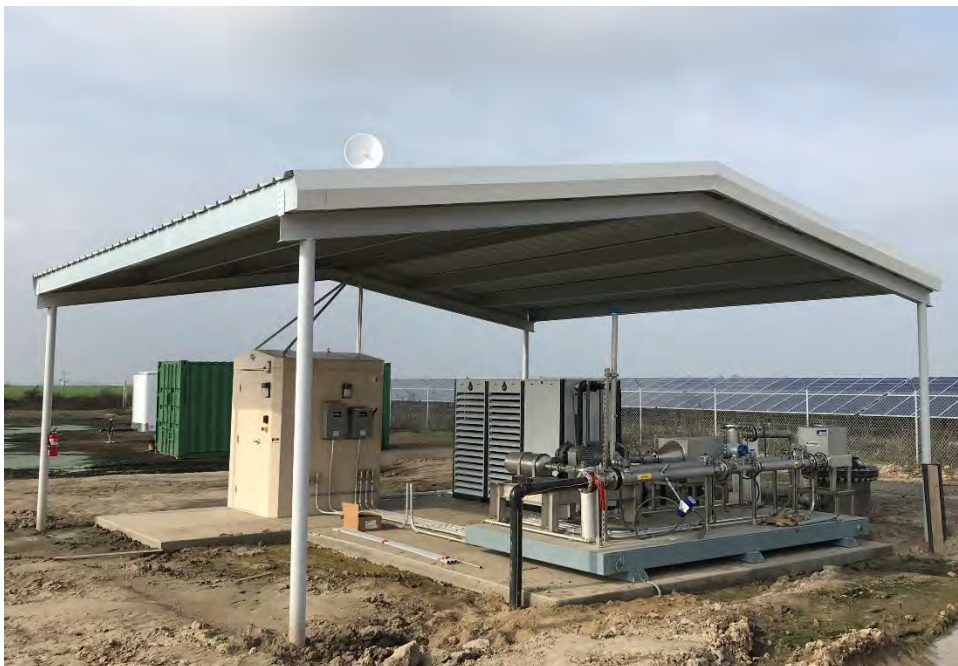
Image 17. Biogas conditioning equipment at Little Rock Dairy.
