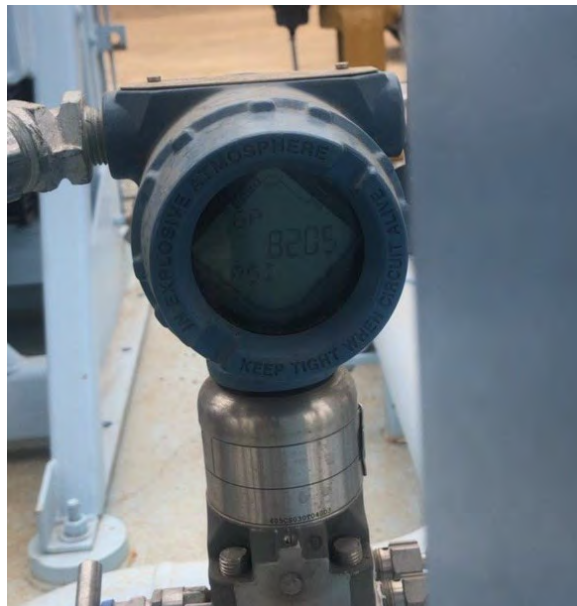
Image 46. Biogas flowmeter at Rancho Teresita Dairy.
