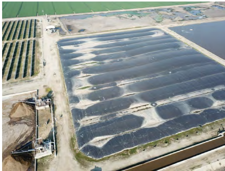
Image 59. New covered lagoon digester at Lakeside Dairy.
