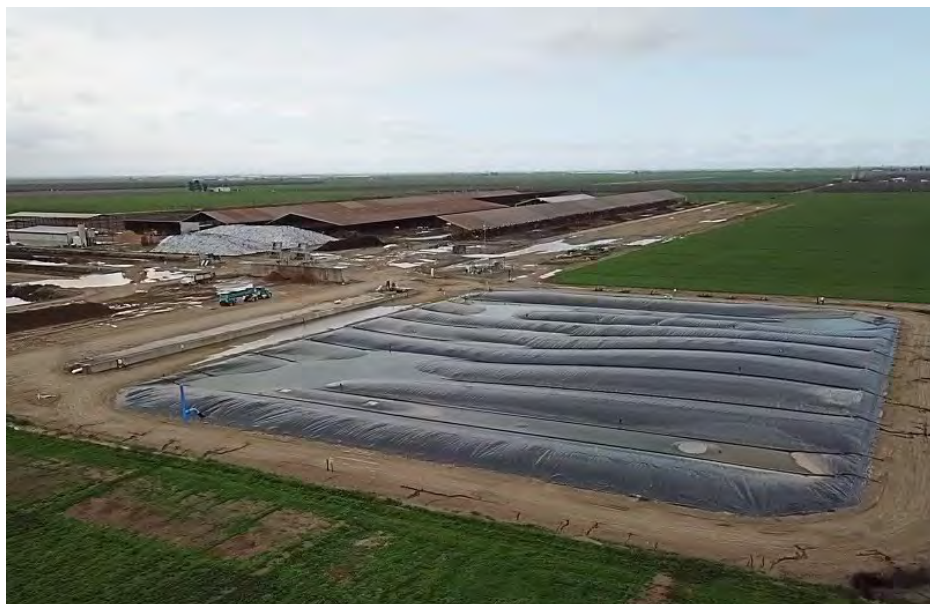
Image 58. New covered lagoon digester at Schott Dairy.
