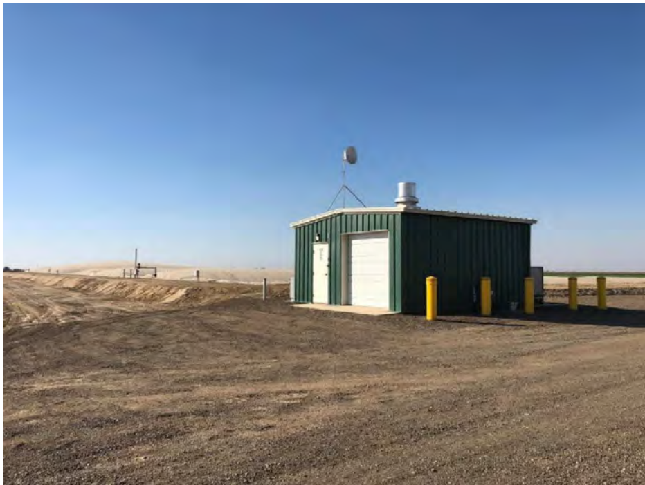
Image 8. View of biogas handling building (foreground) and covered lagoon digester (background) at Circle A Dairy.
