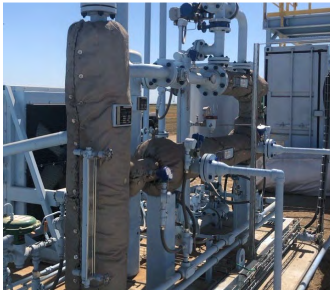
Image 35. Dehydration skid at Dykstra Dairy.
