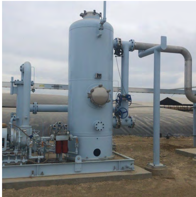
Image 47. Activated carbon vessel at Riverbend Dairy.
