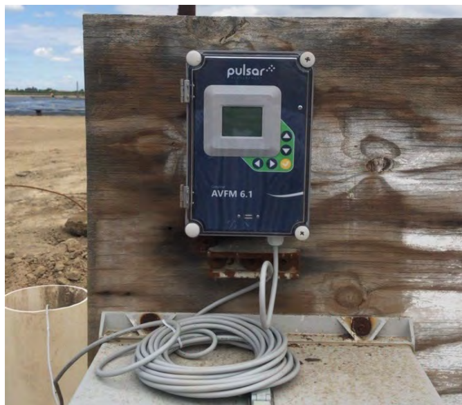
Image 48. Digester wastewater flowmeter at Bos Farms Dairy.
