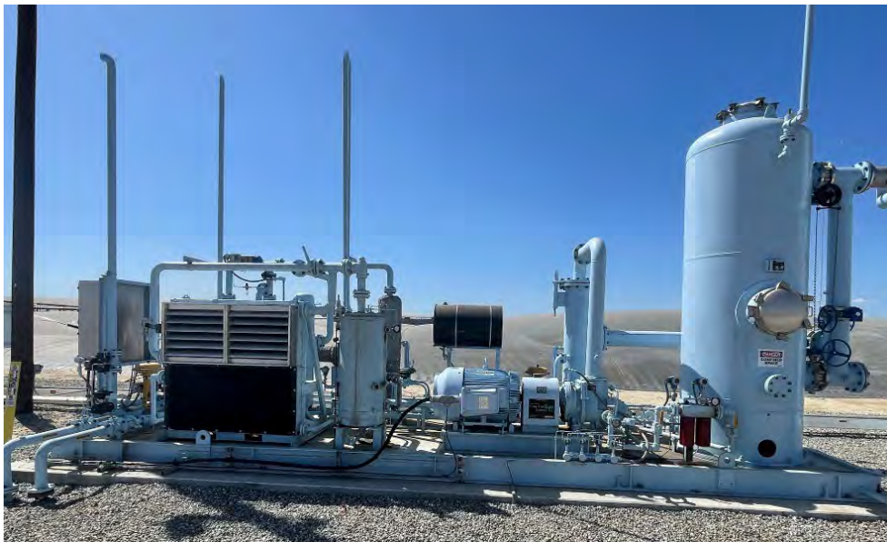
Image 65. Biogas compressor skid equipment at Albert Goyenette Dairy.
