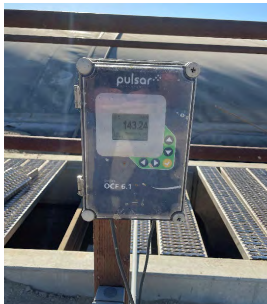
Image 79. Digester wastewater flowmeter at Gerben Leyendekker Dairy.
