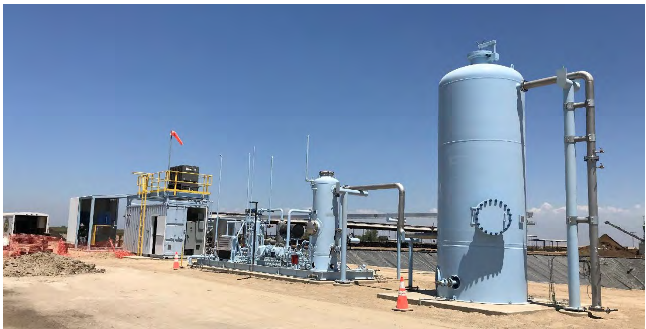
Image 61. Biogas conditioning equipment at Ribeiro Dairy.
