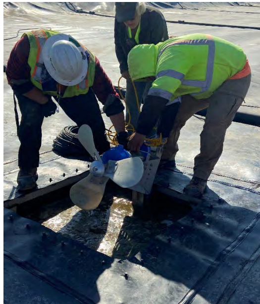
Image 31. Installation of a mixer in the covered lagoon digester at Lone Oak#1 Dairy.
