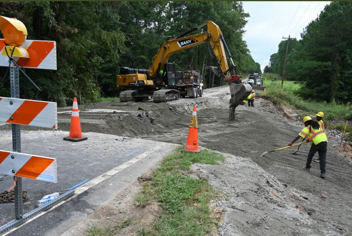
An SCDOT crew works to repair a washed-out section of Dubard Boyle Road in Richland County on August 15.
