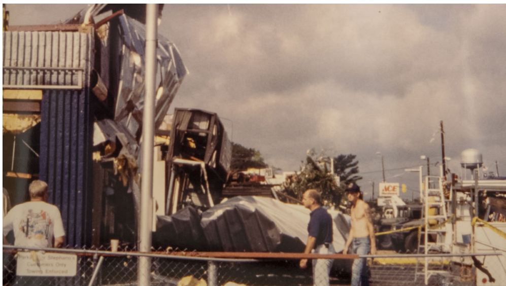
Damage to a building in Lexington caused by an F-3 tornado spawned by Beryl on August 16, 1994 (SCDNR Archive Photo).
