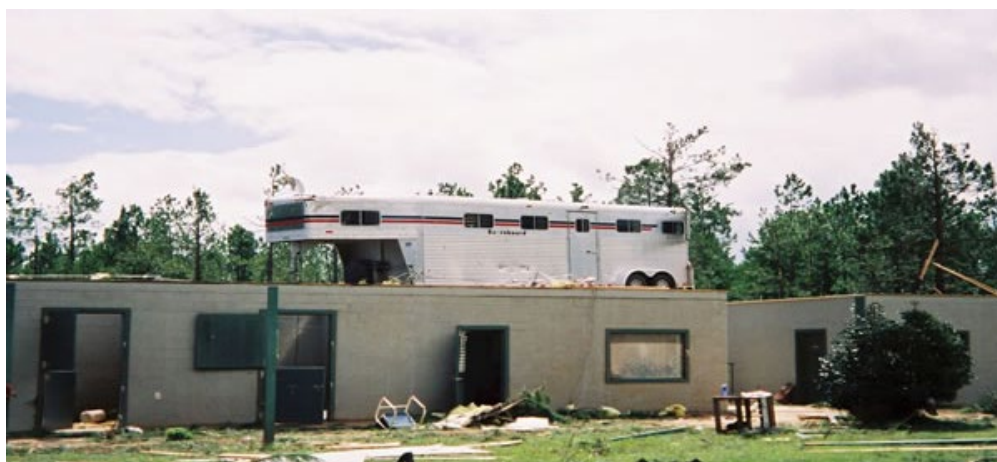
Damage to a horse stable near Camden, with a horse trailer thrown on top of it, caused by the F-3 tornado spawned by Frances on September 7, 2004 (SCDNR Archive Photo).
