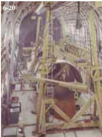
DIAMOND SCULLS underground test facility.
