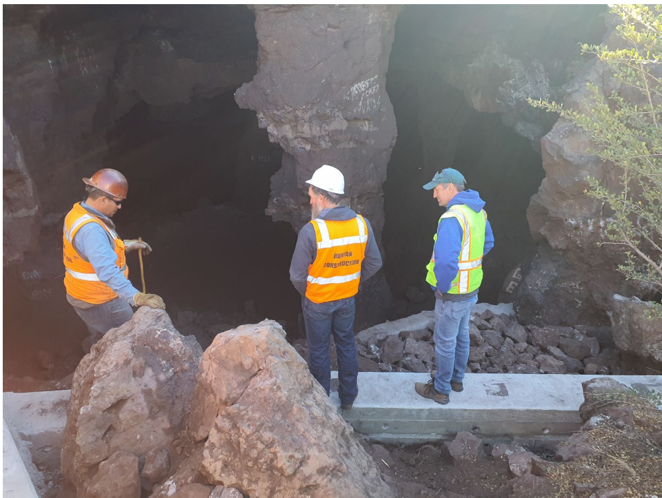
Figure 8: Adit feature LT-134 metal gate closure being measured and cut, the cement base with drainage has been completed.
