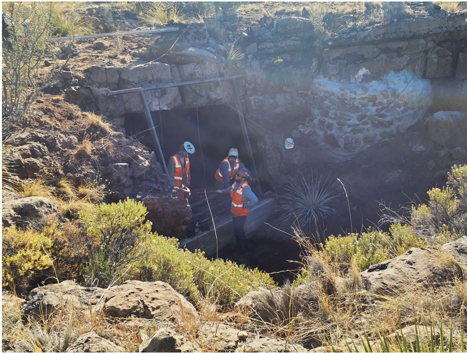
Figure 7: Adit feature LT-8 metal gate closure being erected and adit feature LT-110 waste rock and mortar closure.
