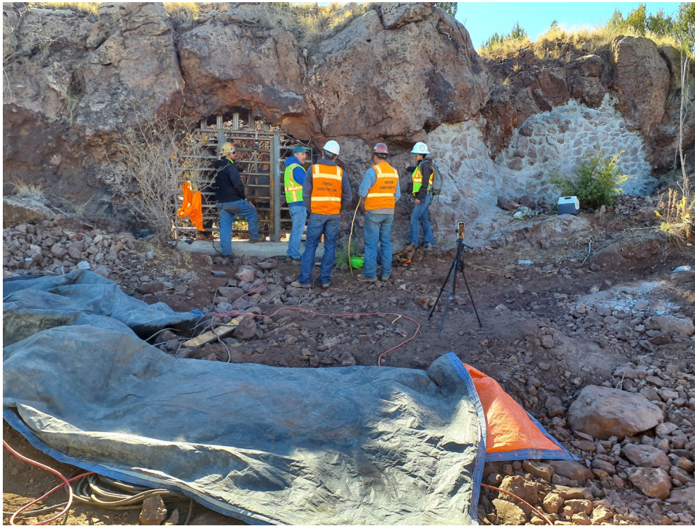
Figure 9: Egress adit feature LT-19 with finished metal gate closure and LT-17 and LT-18 waste rock and mortar closures.
