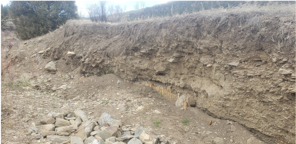
Figure 19. Highly erodible embankment material.
