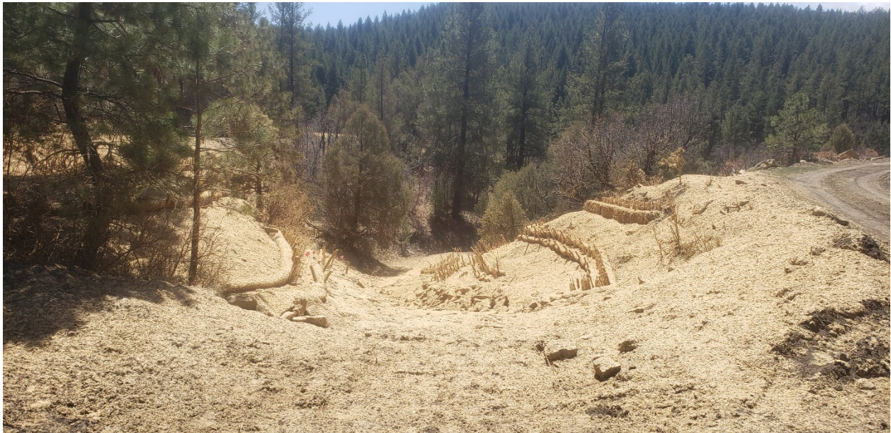
Figure 15. Mulched-over gob piles with coir roll and straw bale terracing and seedlings. Access road center right.
