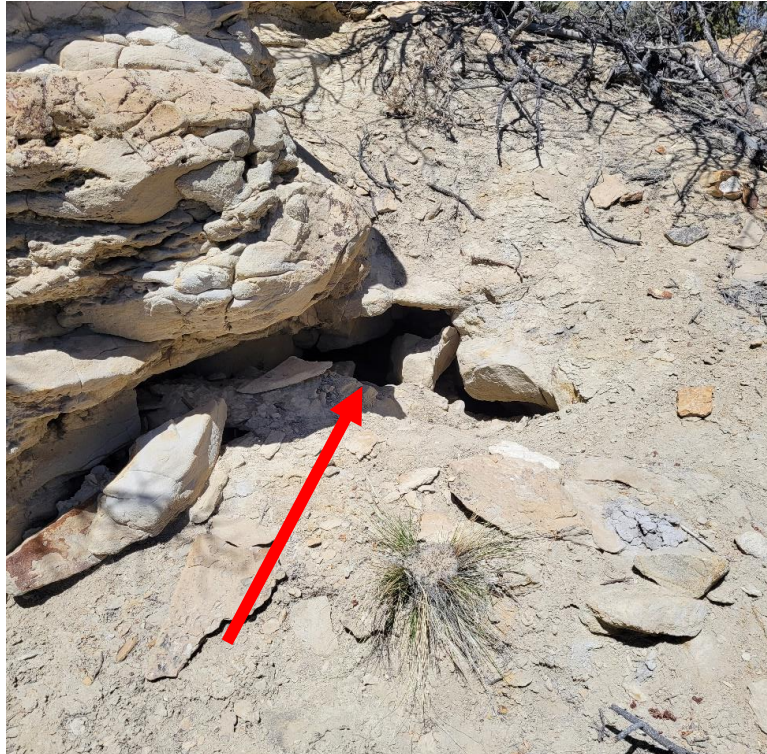
Figure 9: La Ventana Mine Closure Project, Kistler Black Rose Mine, subsidence to the right of feature F-9 (see Figure 7).
