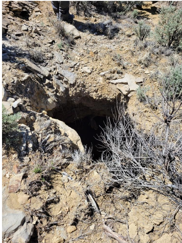
Figure 11: La Ventana Mine Closure Project, Kistler Black Rose Mine, Kistler Black Rose Mine Subsidence.
