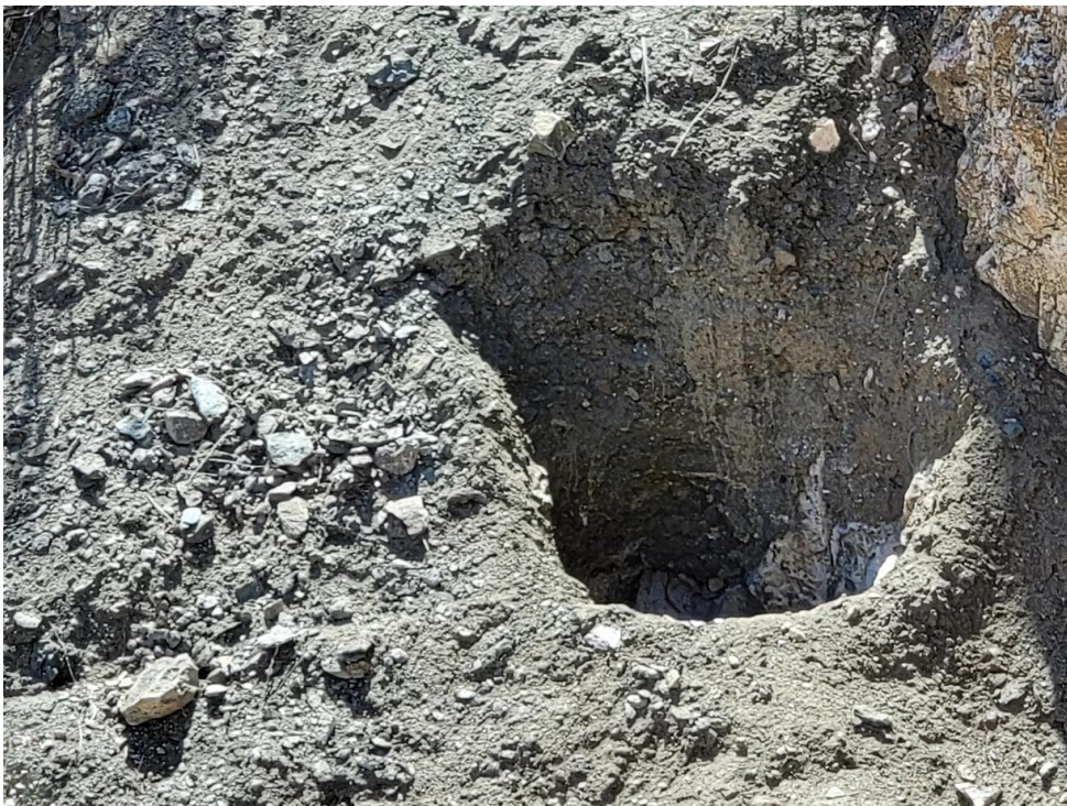
Figure 19: Harding Pegmatite Mine Safeguard Project, S-2 closeup of Subsidence.
