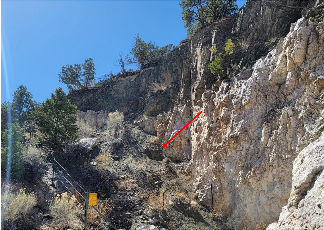
Figure 18: Harding Pegmatite Mine Safeguard Project, S-2 Subsidence.
