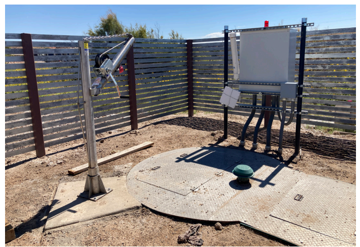
Renovated Lift Station at Lea Lake Recreation Area
