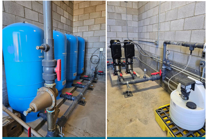
At Left: New pressure tanks At Right: Two new booster pumps and hypo chlorinator
