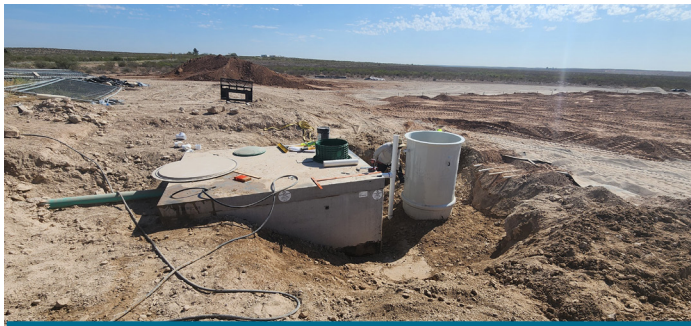
Foreground new 4,000-gal septic tank; background 120 ft by 120 ft evapotranspiration bed, underlain by impermeable liner
