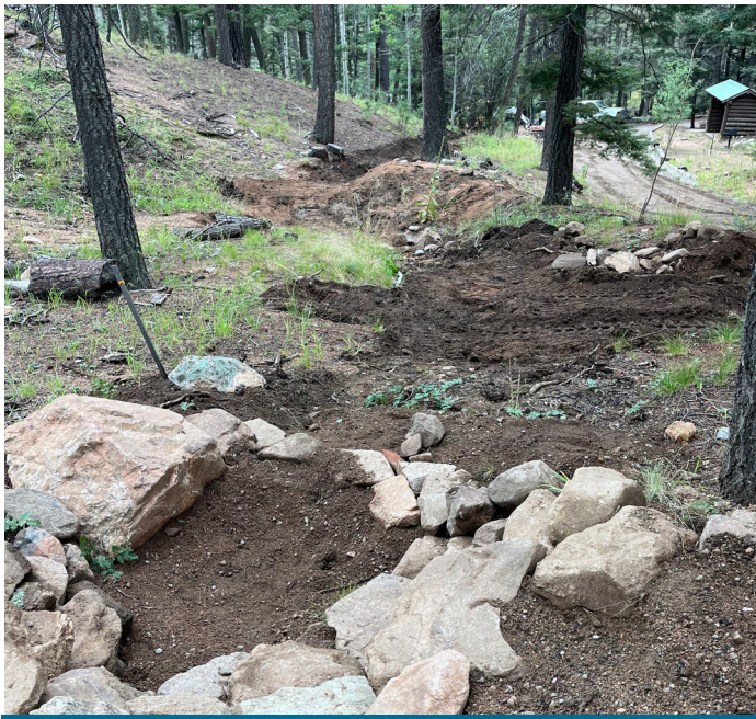
Rock check dams to reduce erosion and increase infiltration of stormwater runoff
