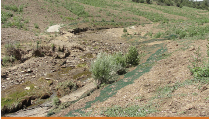
Damage caused by storm in 2013
