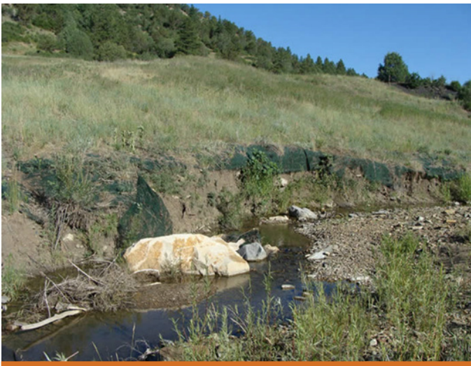
Erosion caused the coal gob material underneath to become exposed
