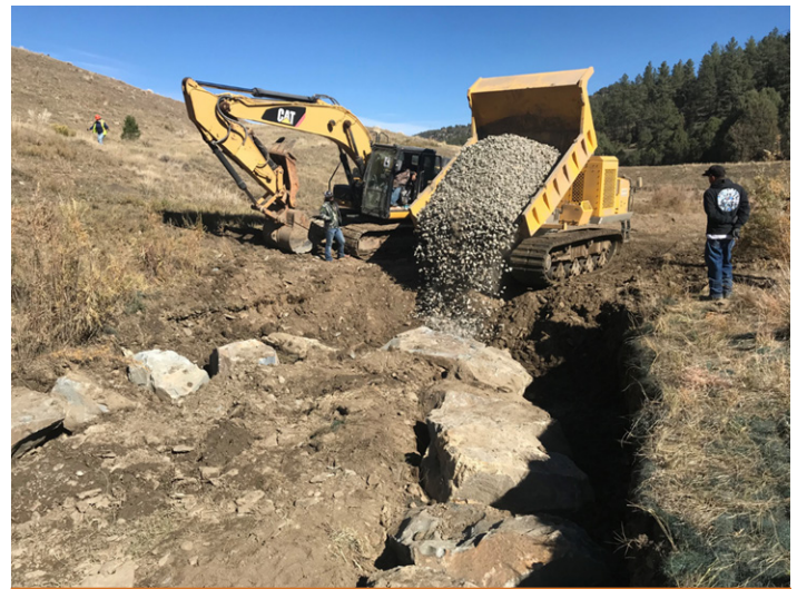
Construction of a cross-vane rock structure at the site, which is an engineered feature designed to create a pool, & slow water flow in the stream channel and prevent erosion.
