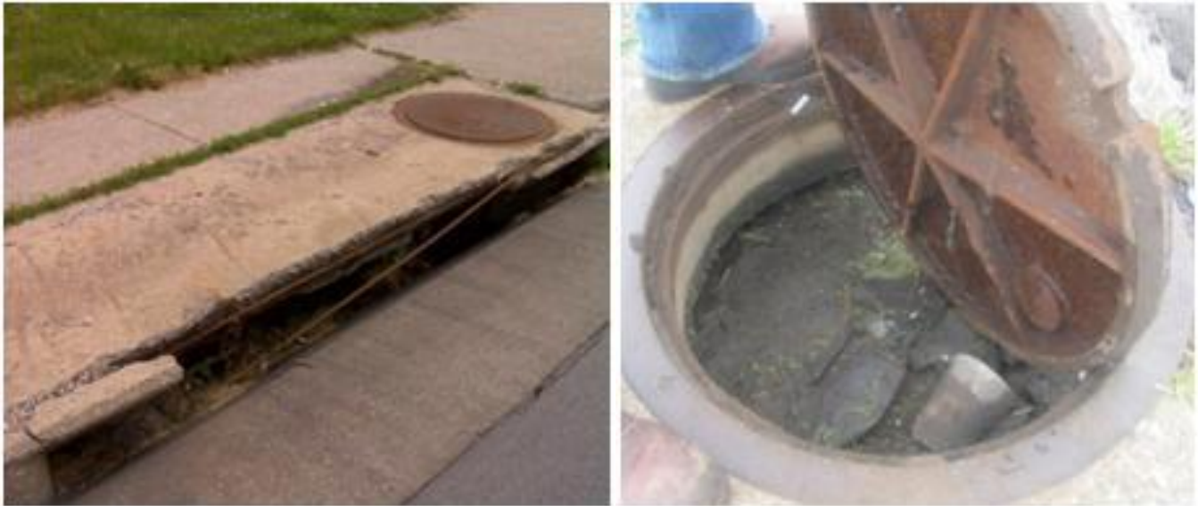
Figure 44. Broken curb inlet; Sediment-filled inlet
