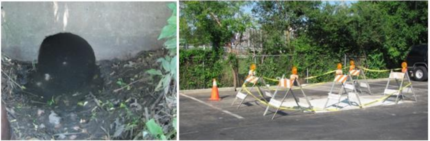
Figure 32. Sewer from line break; Construction on sewer line break
