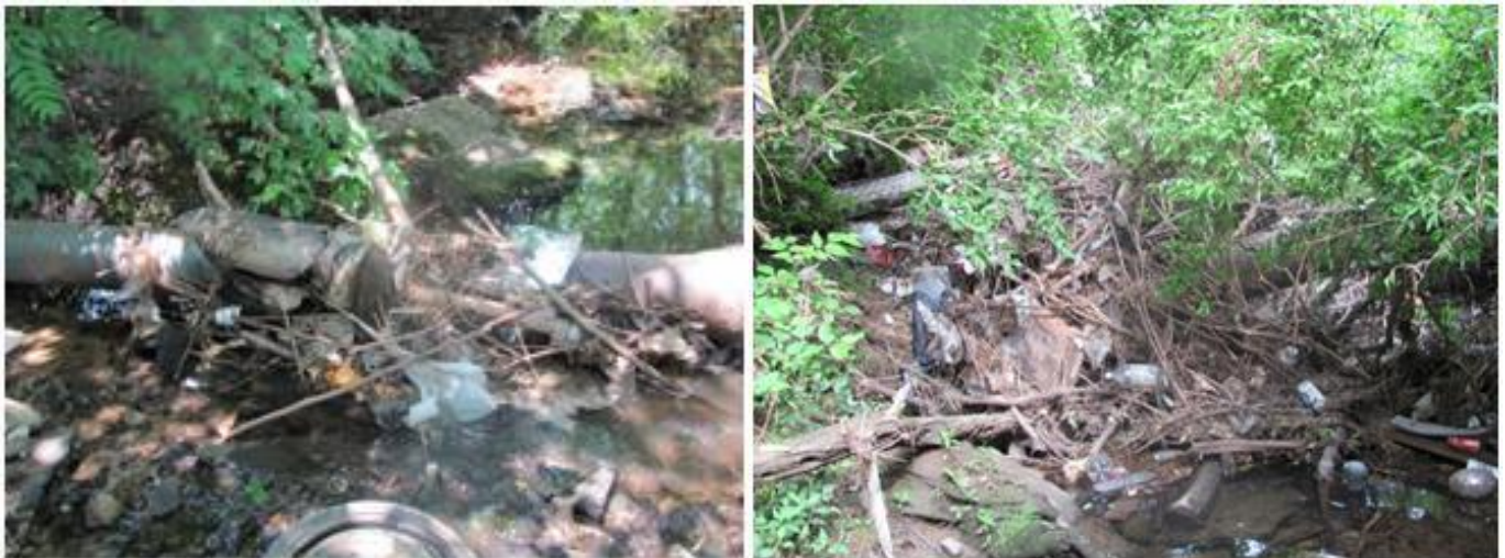
Figure 39. Debris clogging around pipes; Possible area for LFUCG and UK Fusion Cleanups
