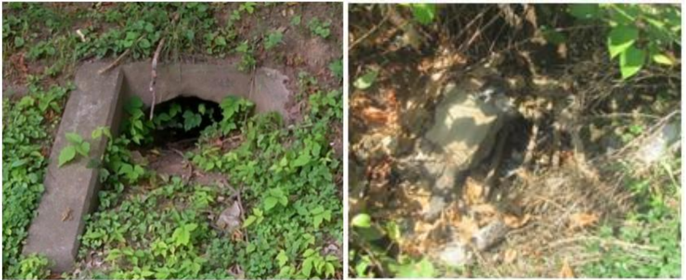
Figure 29. Endwall filled with mud and vegetation; Endwall filled with trash and debris
