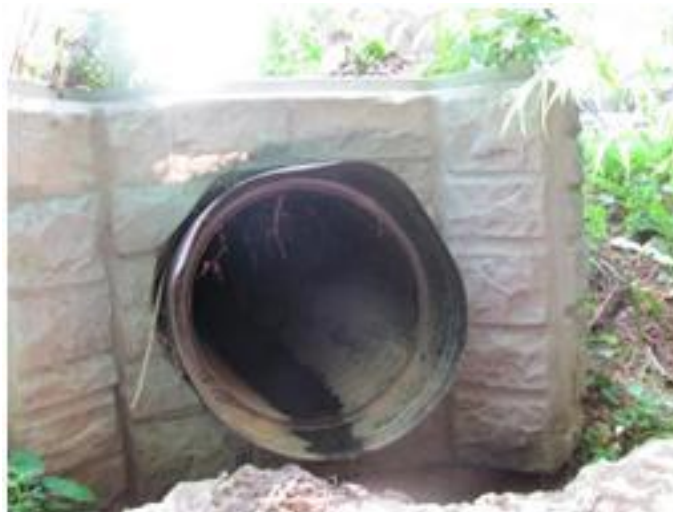
Figure 33. Faux rock endwall
