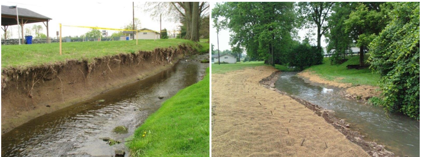
Figure 78. Cane Run tributary before Lexmark restoration; Cane Run tributary after Lexmark restoration
