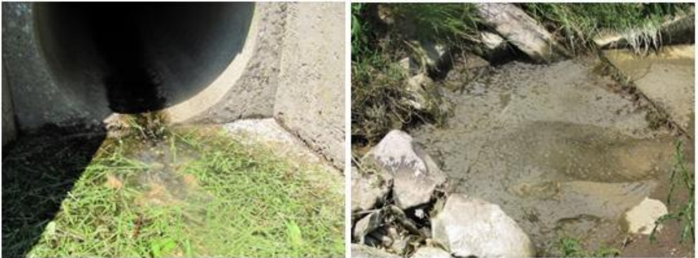
Figure 31. Brown liquid discharging from endwall; Sudsy water discharging from endwall
