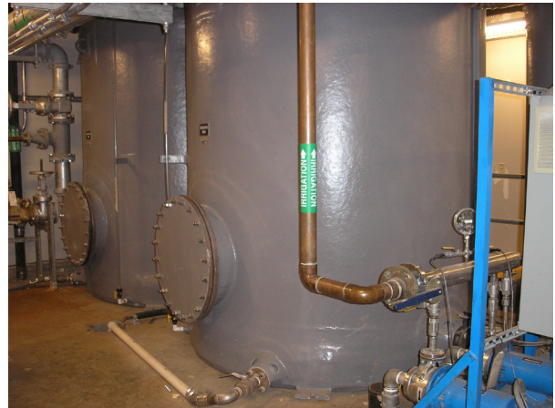
Two 2,500-gallon tanks storing air handler condensate and harvested rainwater for irrigation
