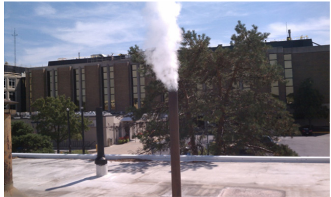
Figure 10. Example of steam plume from a roof vent, indicating a failed steam trap.
