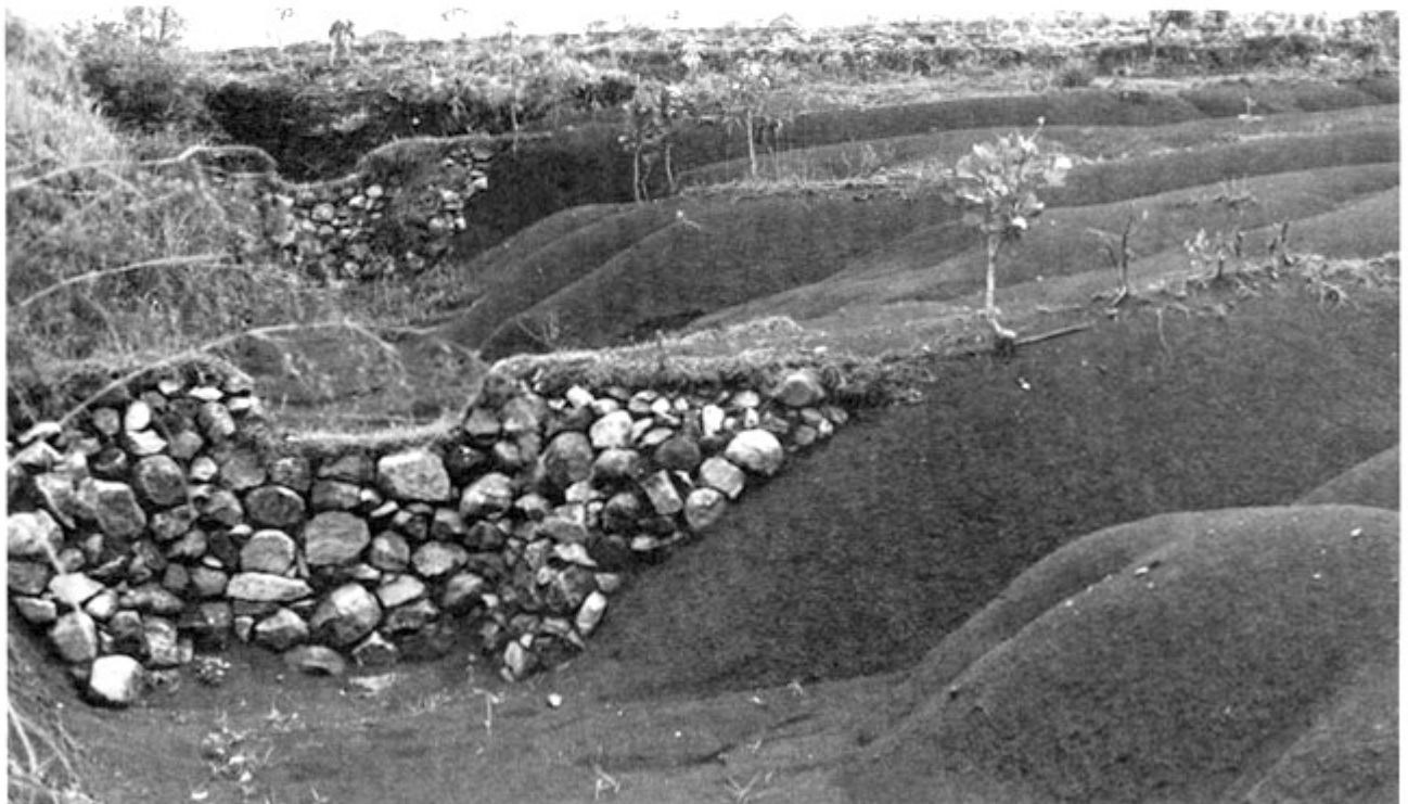
Fig. 100 Check dams in gully. Silt settles behind the dams, thus filling the gully, enabling terrace construction and rehabilitation of a critically eroded area in the Upper Solo Valley, Indonesia (WFP photo, issued by FAO)
