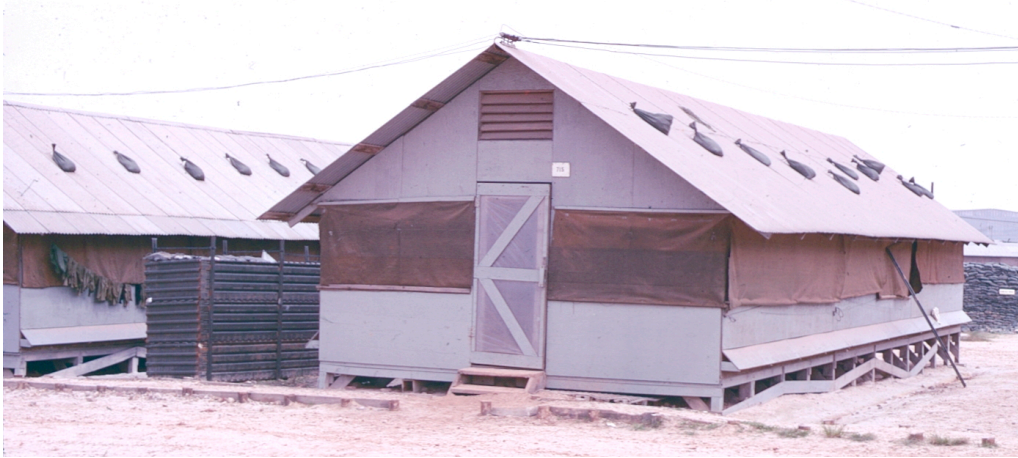
I think this is my hooch ... note the “blast wall” to the left.
