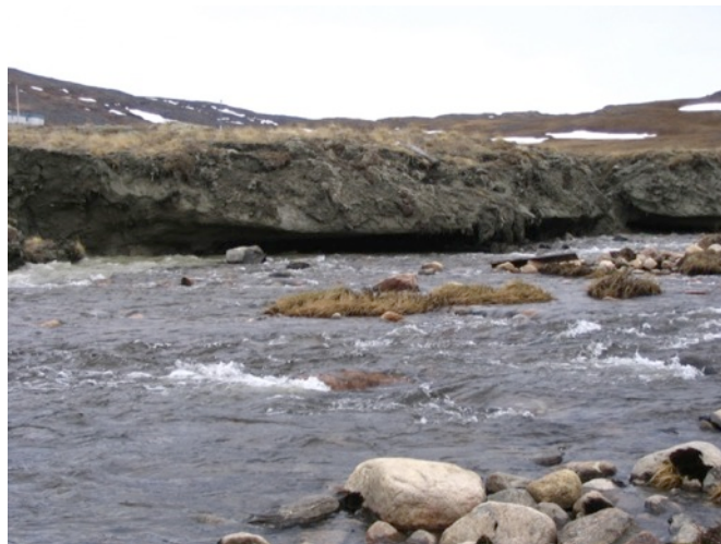
Figure 23. The extreme peak discharge of the Duval River in June 2008 resulted in the downcutting of the river bed, caused thermo-erosion and the collapse of the Hamlet's bridges (Photos Michel Allard's team).
