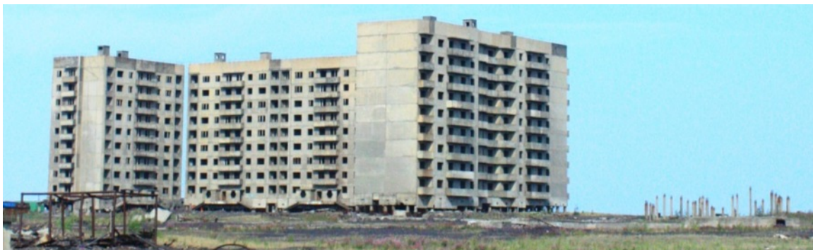
Figure 29. Building constructed using piling foundation on permafrost. The same type of piles can be seen on the right from the building. Various heights of the piles are the result of differential frost heave processes over the construction site. (Photo: D. Streletskiy, July 2013)
