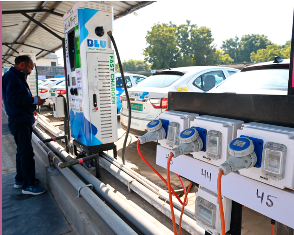
India's largest EV charging station in Gurugram, the business capital of Haryana. SOURCE: Sudarshan Jha via Shutterstock
