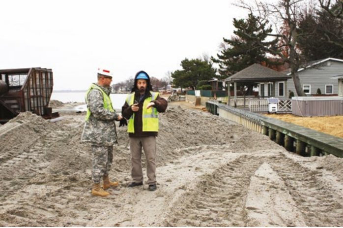
U.S. Army Corps of Engineers discuss plans to build a berm in Oakwood Beach to protect against future storm damage. Source: USACE, Flickr/CC (2014).
