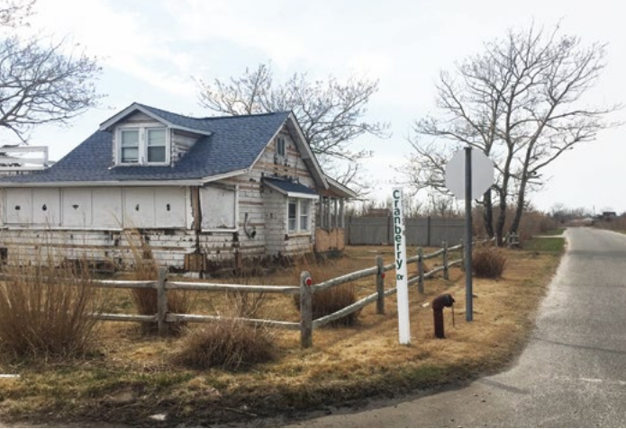
This Mastic Beach home was vacated after it was damaged by severe flooding. Source: Regional Plan Association.
