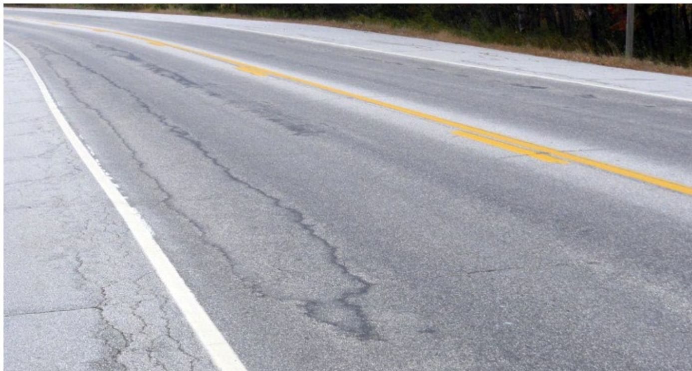
Figure 2 - Example of severe HMA erosion through surface into underlying layer
