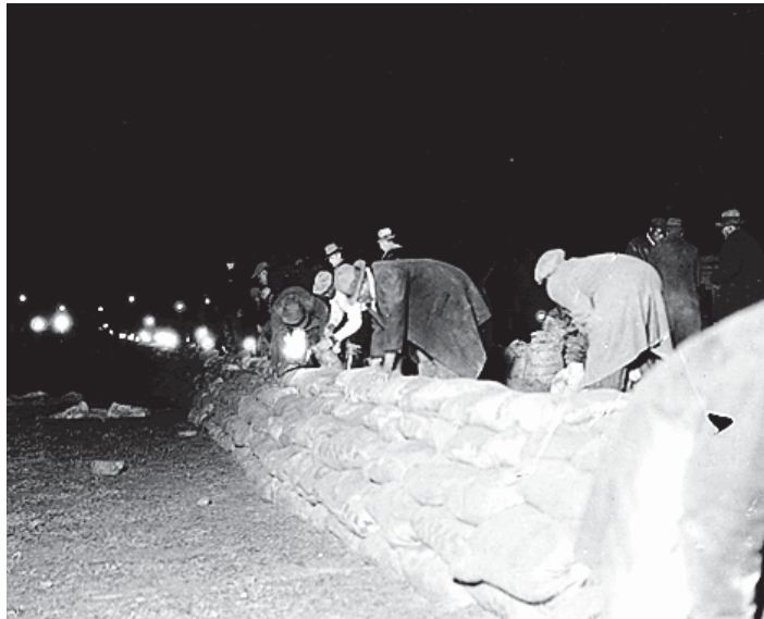
Workmen from the Works Progress Administration (WPA) use sandbags to build an emergency levee against the Great Spring Flood of 1936 in Washington, D.C., the event that led Congress to order the building of a permanent levee along the National Mall. PHOTO, DEPARTMENT OF THE INTERIOR
