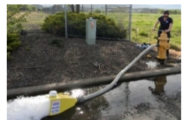
Routine maintenance such as hydrant operation and flushing helps ensure water quality from the source to your tap.
