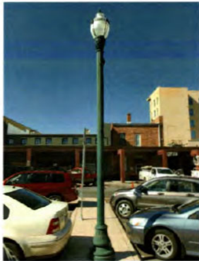
Fig. 6 Example of Cultural District Green Decorative Pole with Period Light
