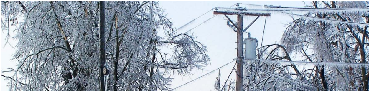
Figure 2: Frozen power lines
