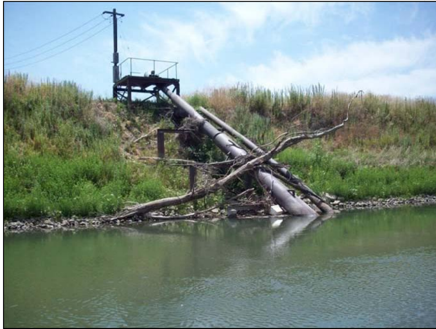
Figure 67. The Windswept pump station intake looking in a downstream direction.
