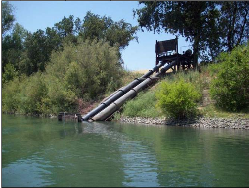
Figure 15. The Sycamore pump intakes looking in a downstream direction.
