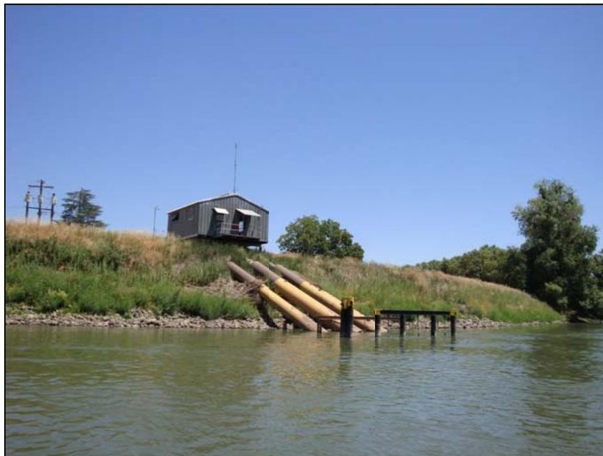
Figure 78. The Portuguese Bend pump station intakes looking in a downstream direction.
