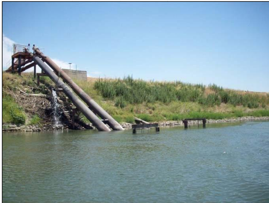
Figure 59. The Oji pump station intakes looking in a downstream direction.
