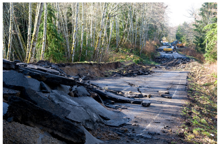
State Route 112 in Sekiu, WA suffered severe damage from flooding in the aftermath of storms in 2009.
